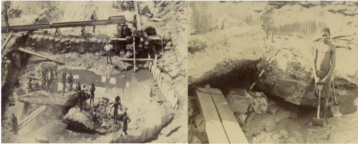
Picture 8: Black workers under white supervision constructing new footings for the flooded Kaap River Bridge; Picture 9: Black African labourer preparing the river bed for the construction of new footings for the Kaap River Bridge 197
