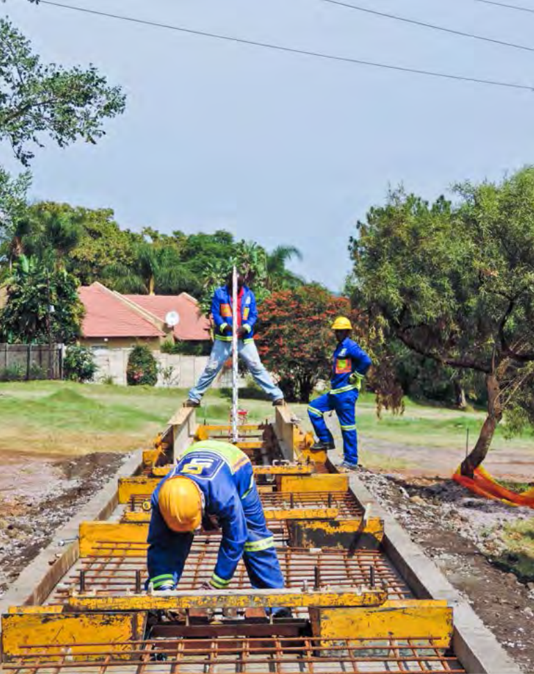
Construction of the PY Slab Track test section for the University of Pretoria
