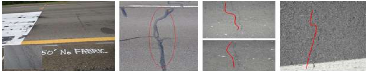
Fig. 3a. Existing Highway US 59 Pavement Condition Prior to HMA Overlay Construction.
