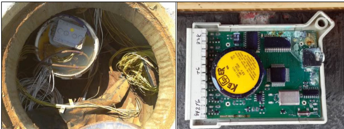
Figure 4-2: Flooded manhole and water-damaged Smartreader unit (Steyn and Coetzer, 2015).
