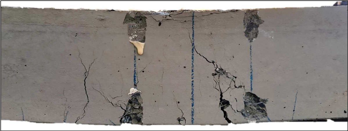
Figure B. 33: Crack formation along left span after testing
