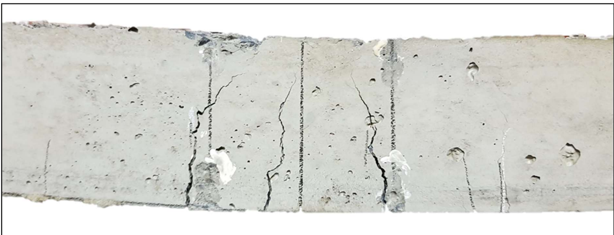
Figure B. 4: Cracked section at right span after testing
