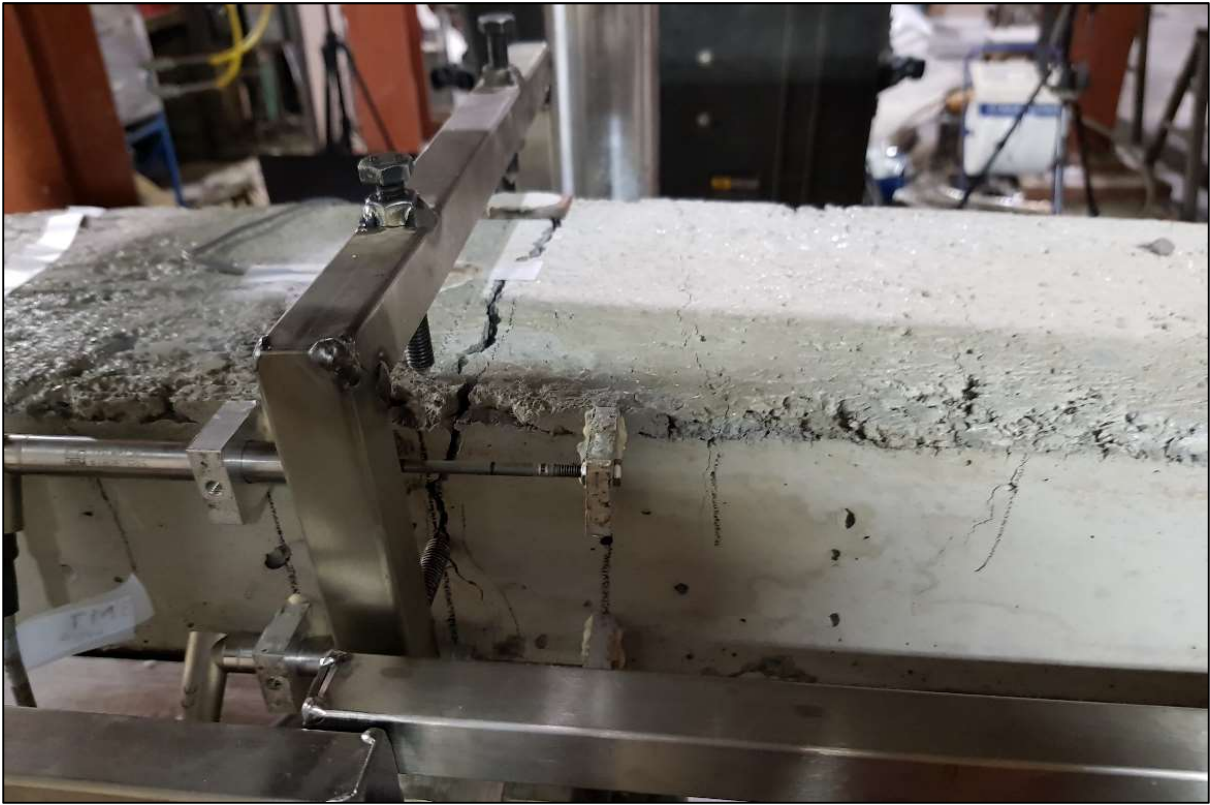
Figure B. 3: Cracked section at centre support
