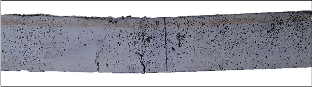
Figure B. 7: Cracked right span after testing
