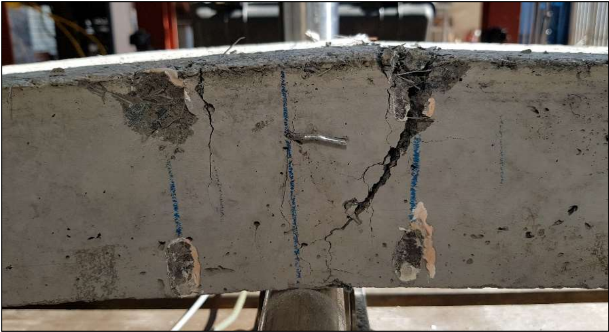
Figure B. 21: Cracking above centre support after testing
