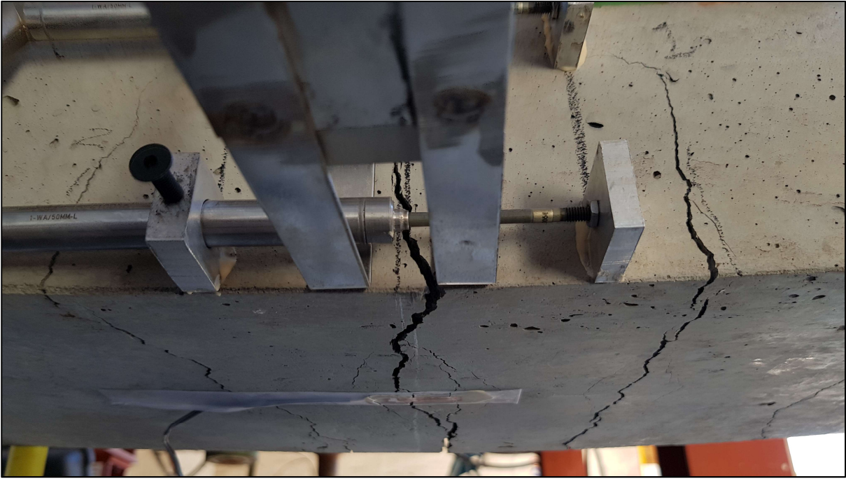
Figure B. 2: Cracked section under left span
