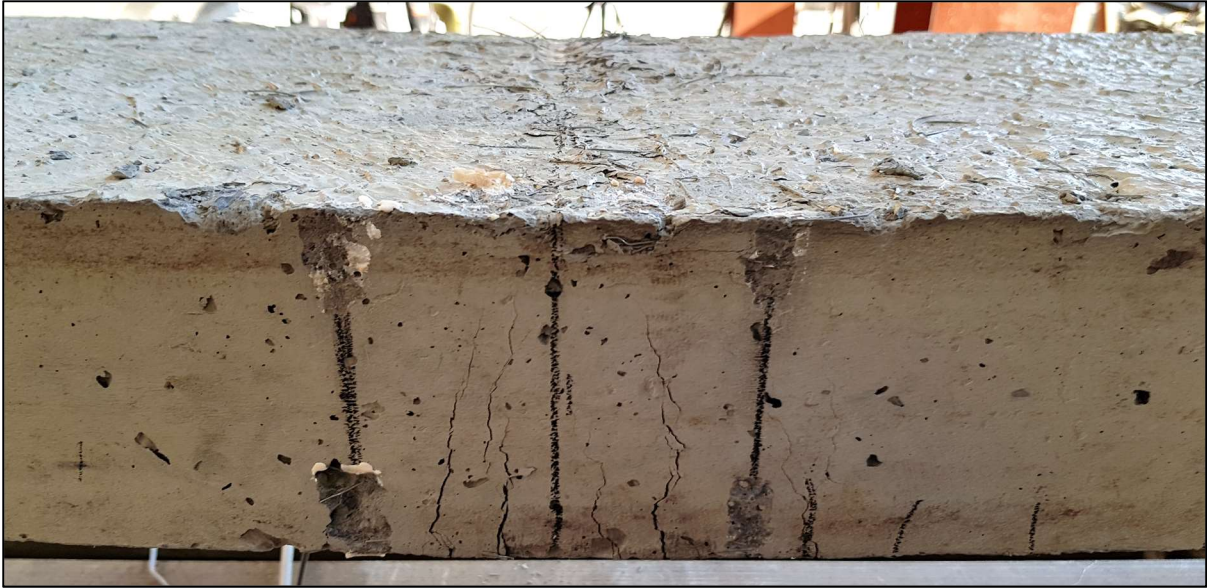
Figure B. 13: Cracks at left span after testing
