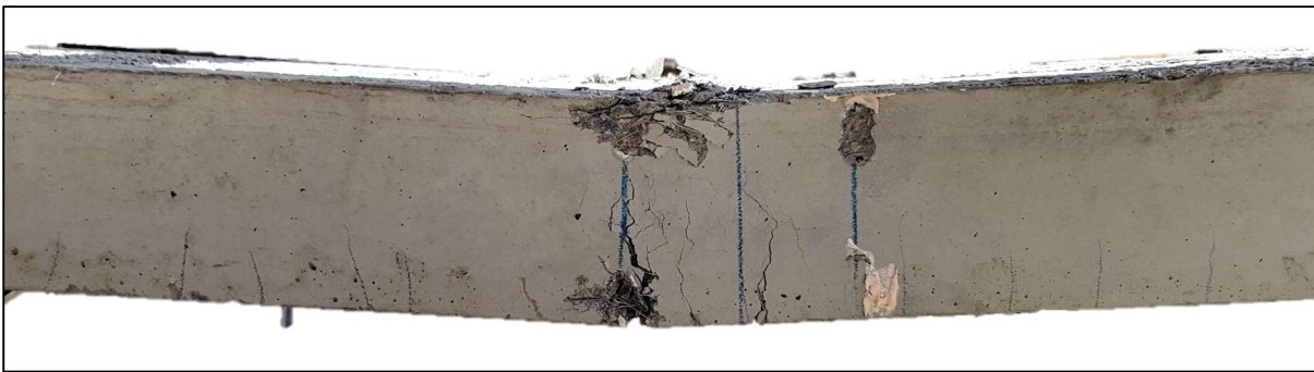
Figure B. 22: Crack formation of left span after testing
