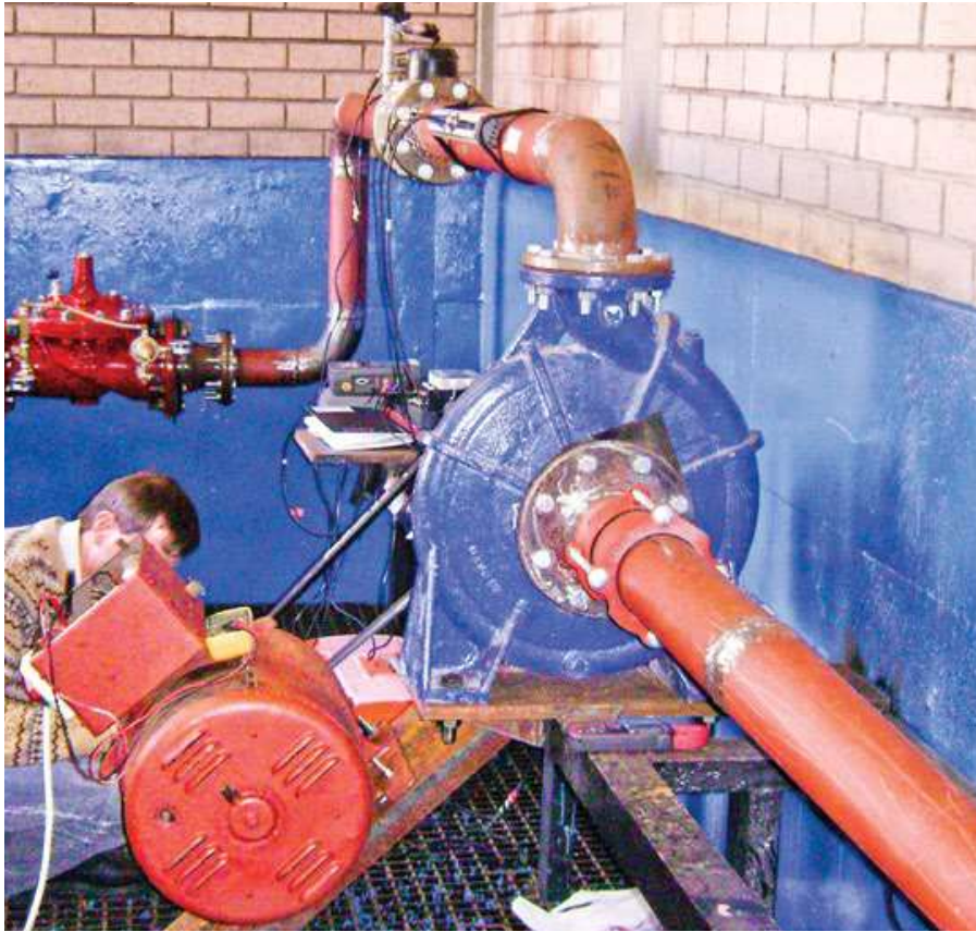
Figure-6 – PAT installation – Queenswood Reservoir – City of Tshwane, South Africa (Loots et al., 2014)
