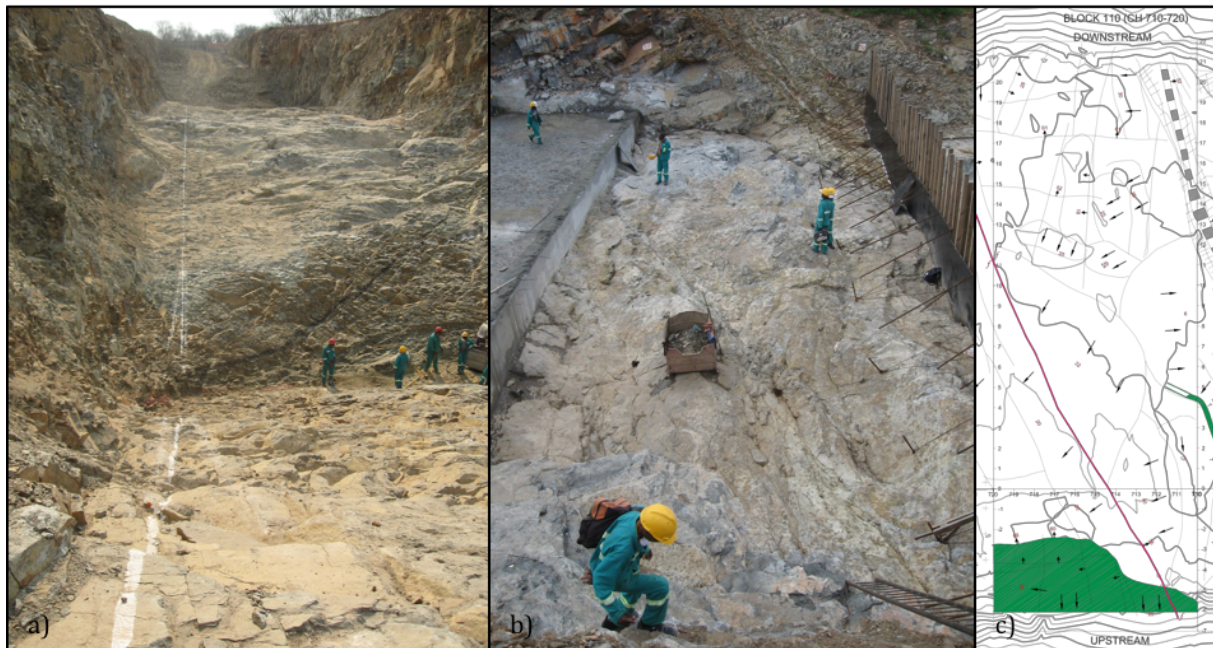
Figure 5-2 Foundation excavation at De Hoop Dam: a) dam wall axis at the left flank; b) cleaned foundation block ready for detailed geological mapping before concrete placement; and c) as-built geological plan of the respective block (photographs and drawing courtesy of Knight Piésold).
