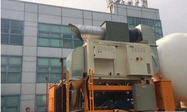
(b) Emission control unit on
