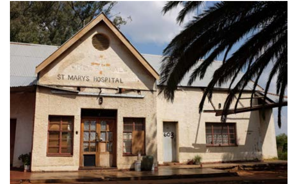
Figure 3-18: Deterioration of building (Clarke 2014)
