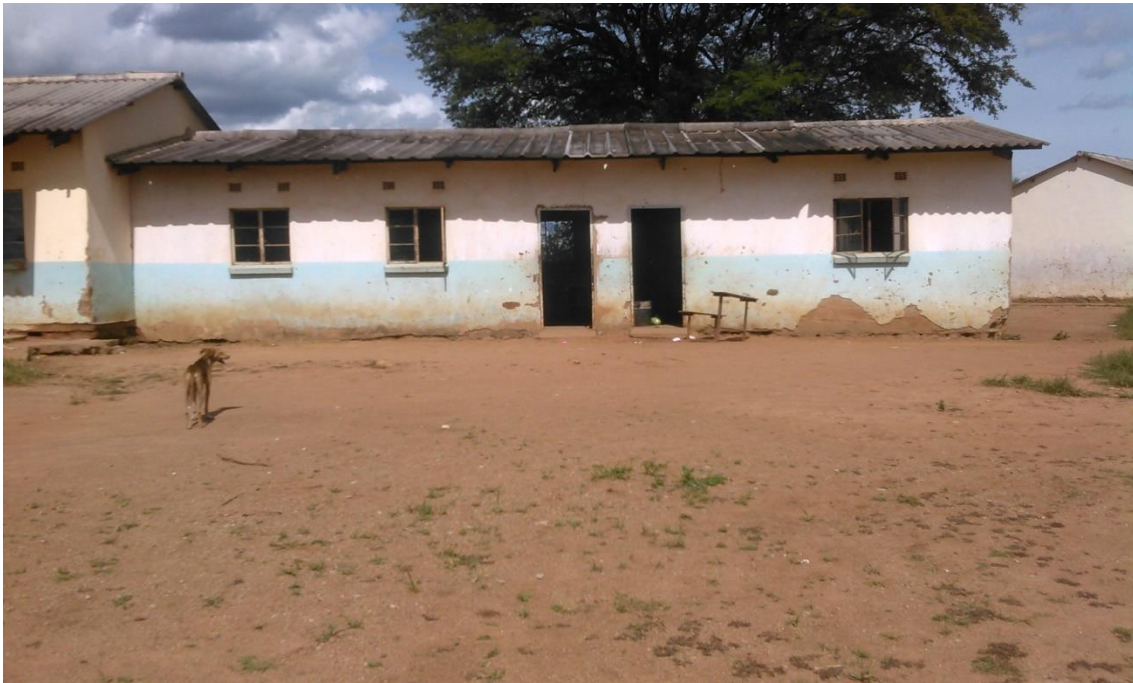
Figure 4: A classroom-block awaiting renovation at Mugoto Basic School
