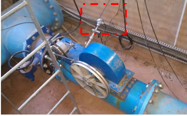
Figure 3-6: RTD installed at Pierre van Ryneveld reservoir
