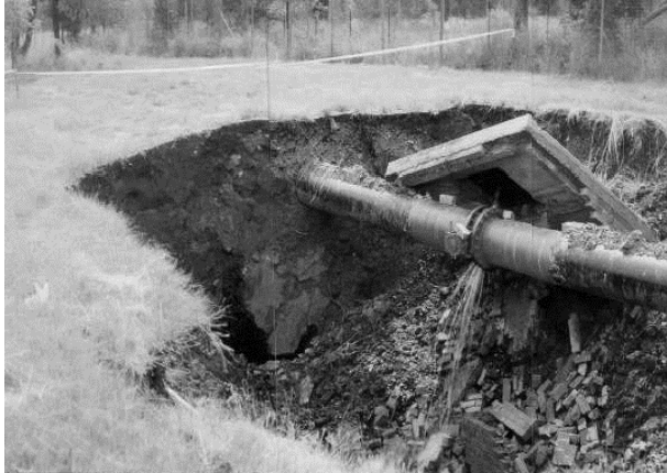
Figure 2-7: Leaking water pipe caused a sinkhole to form Pretoria (Oosthuizen and Richardson, 2011)
