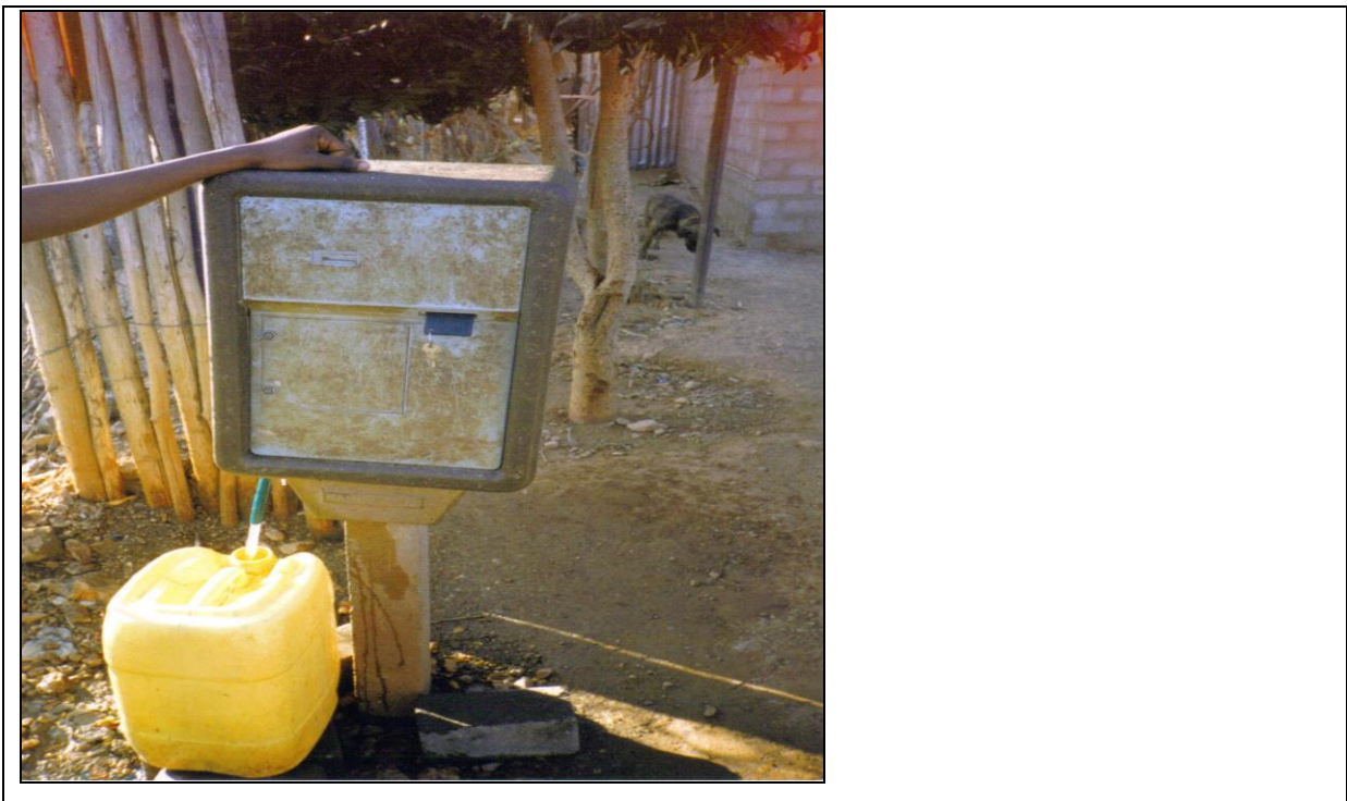
Figure 1: Prepaid Water Meter System
