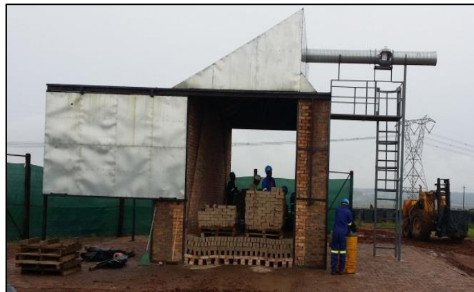
Figure 1: Ongoing model kiln packing process showing horizontal stack, sliding door enclosures, sampling platform and green mesh windshield
