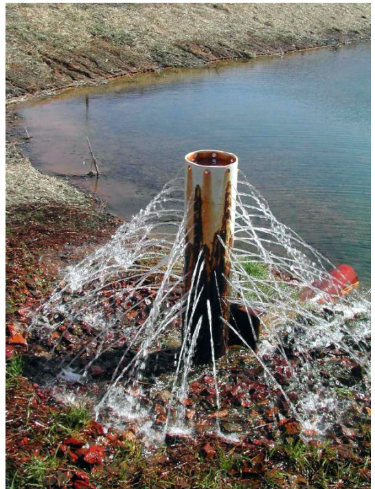
Figure5. 12 Aeration pipe at the Vintondale AMD&ARTS park's pond 6 (AMD&ART 2016)
