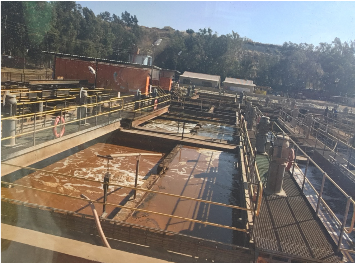
Figure 8.50 AMD treatment facility in West Rand (Author 2017)
