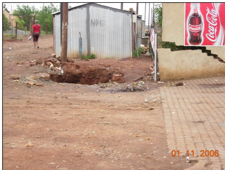
Plate D.1: Sinkhole and subsidence in area of Borehole BH8.
