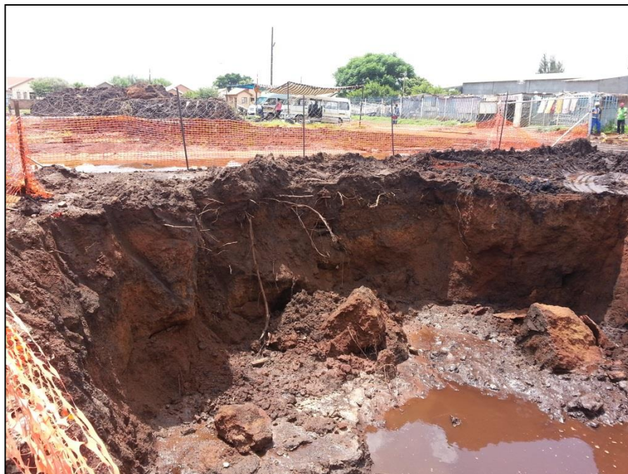
Plate C.1: Bulk excavation in progress below water level causing unstable side slopes and collapse.
