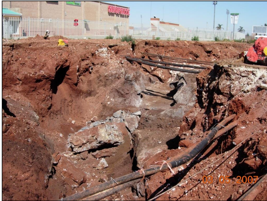
Plate F.3: Photo of gryke taken towards the south with soft rock dolomite capping removed over cavity in area of east-west aligned cables.
