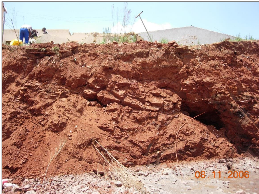
Plate D.2: Cavity exposed during bulk excavation in area of Borehole BH5.
