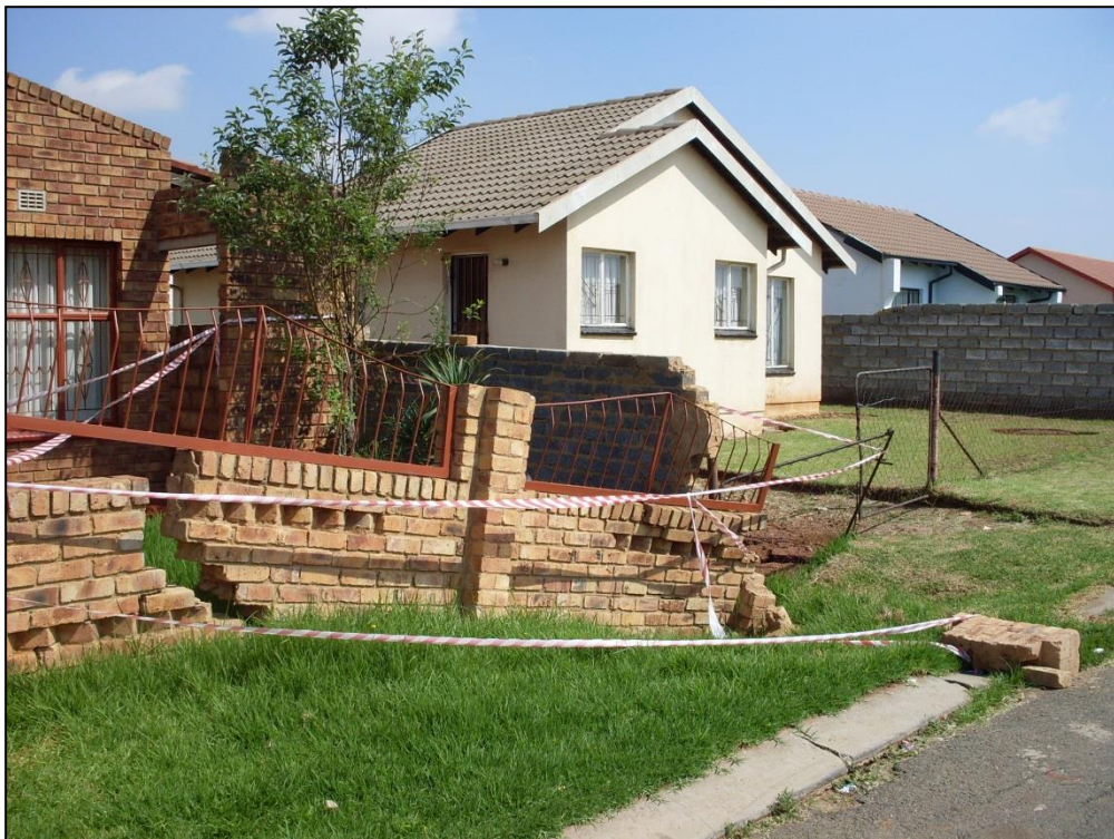
Plate B.1: Sinkhole on eastern boundary of Stands 1063 and 1064, Njakata Crescent Street, Vosloorus Extension 2.
