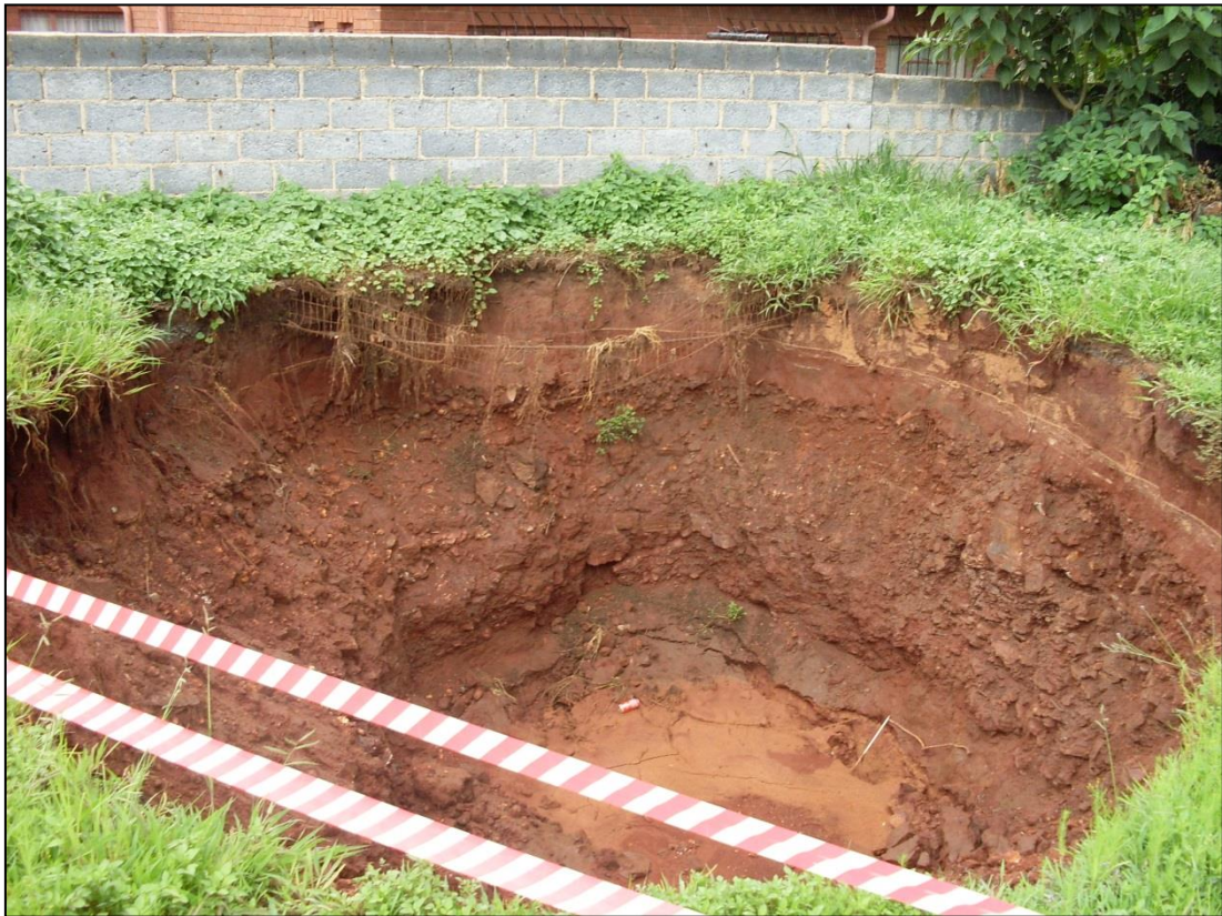
Plate J.1: Sinkhole on Stand 2, Tembisa, photo taken towards the west.
