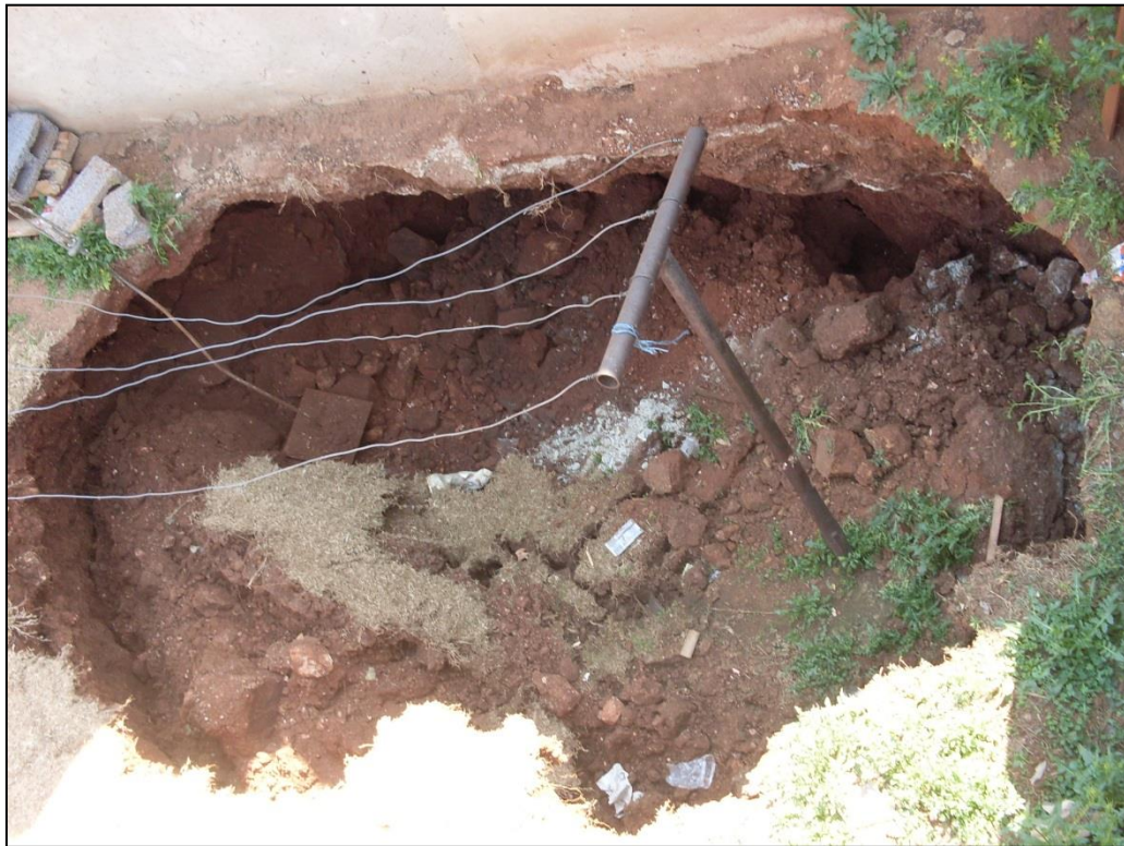
Plate I.2: Close-up view of sinkhole on Stand 20121 Vosloorus Extension 30.
