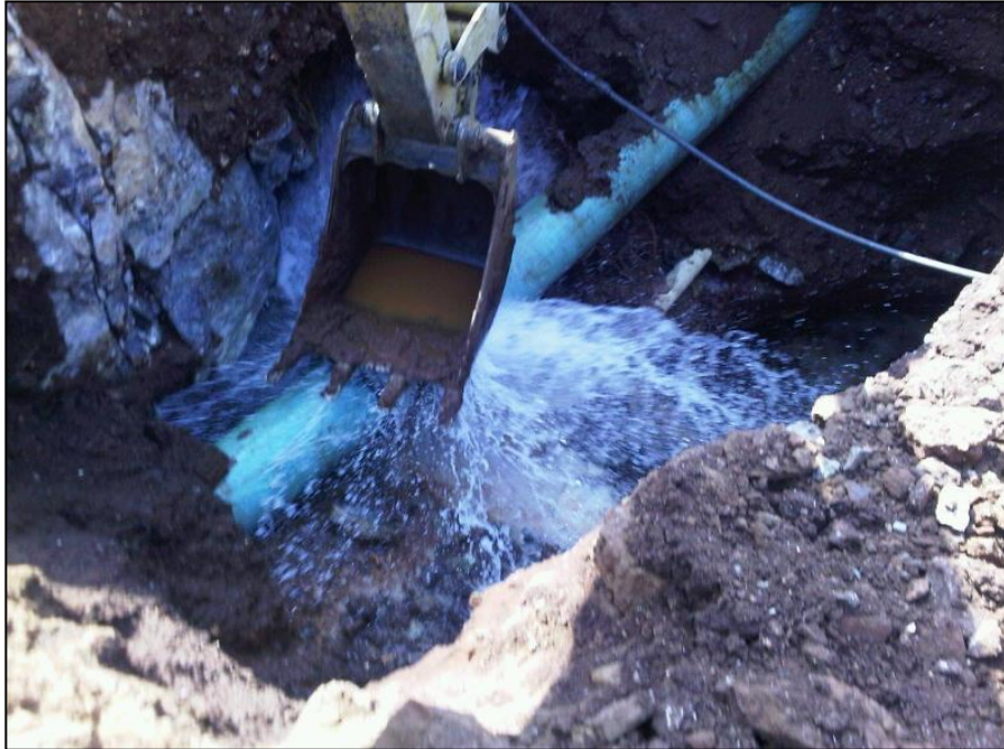
Plate H.1: Water from broken water line disappearing along a subsurface erosion tunnel in a northerly direction.
