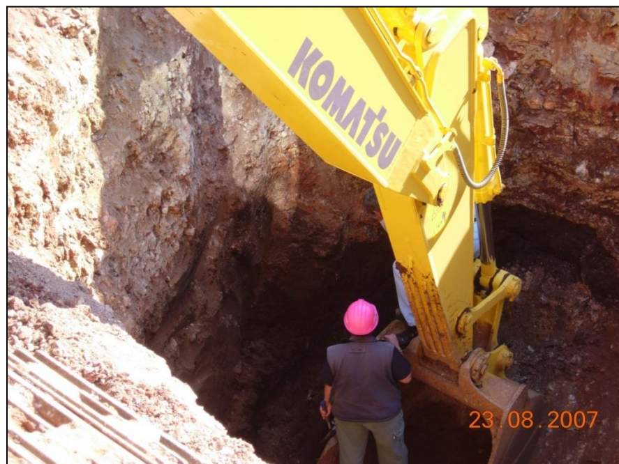
Plate E.4: Cavity exposed during bulk excavation of sewer and sinkhole north-west of Stand 2636.
