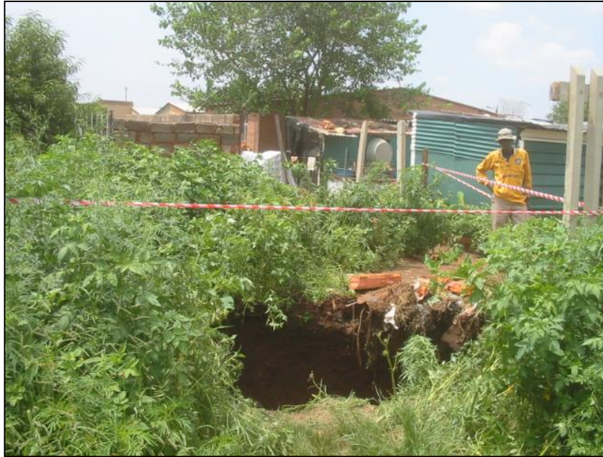
Plate E.3: Sinkhole at north-western boundary of Stand 2656.
