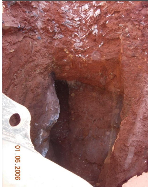
Plate A.5: Exposure of erosion tunnel in southern side wall of Bierman Road excavation.
