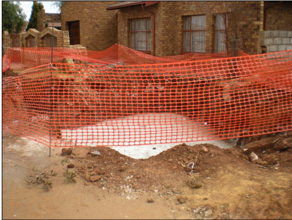
Plate B.2: Bulk excavated area and cavity backfilled with 10 MPa mass concrete.
