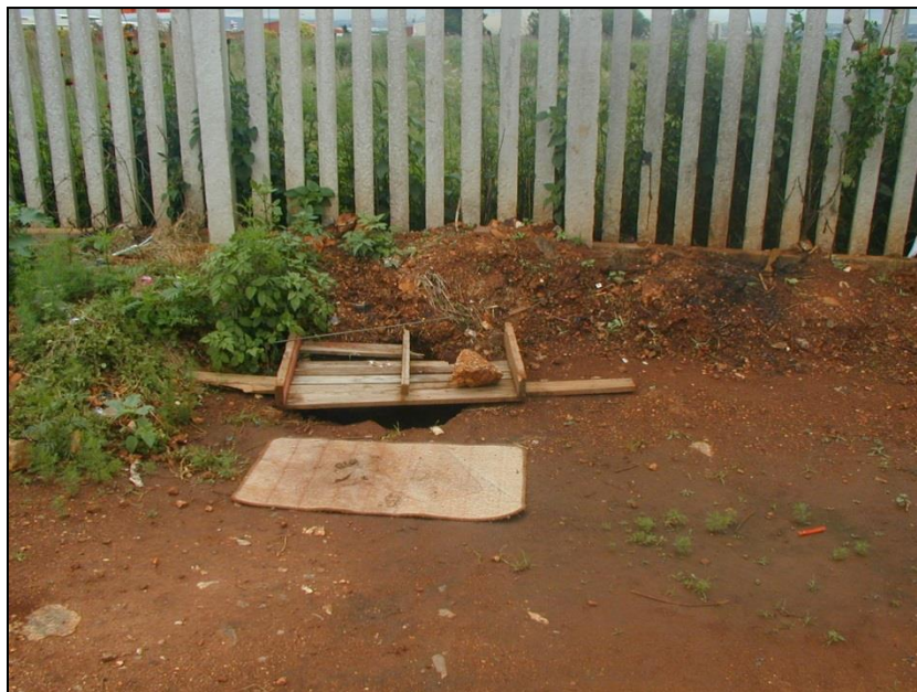
Plate E.1: Sinkhole on western boundary of Stand 2636. A sewer manhole is situated 18 m north-east of the sinkhole.
