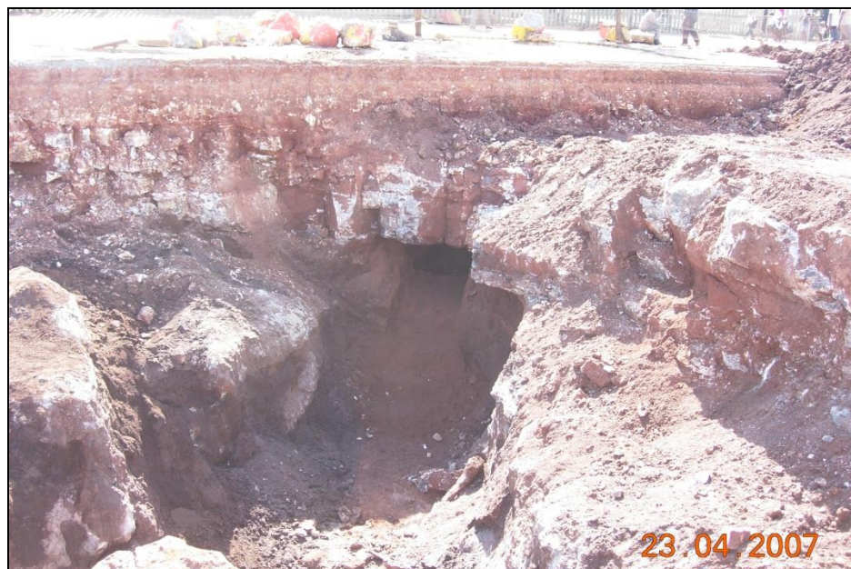
Plate F.5: Cavity exposed in northern corner of bulk excavation area with soft rock chert roof.
