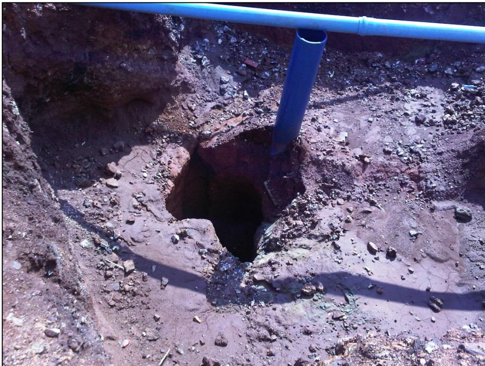
Plate G.1: Sinkhole in trench excavation for a proposed water line.
