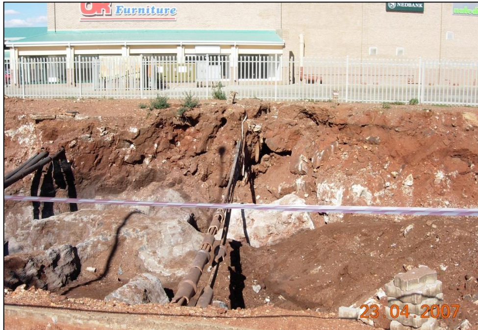
Plate F.4: Soft rock dolomite roof over a 1 m high and 10 m diameter cavity.
