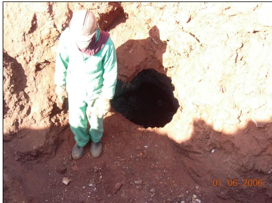
Plate A.2: Cavity encountered in Borehole BH2 and at base of sewer trench excavation.
