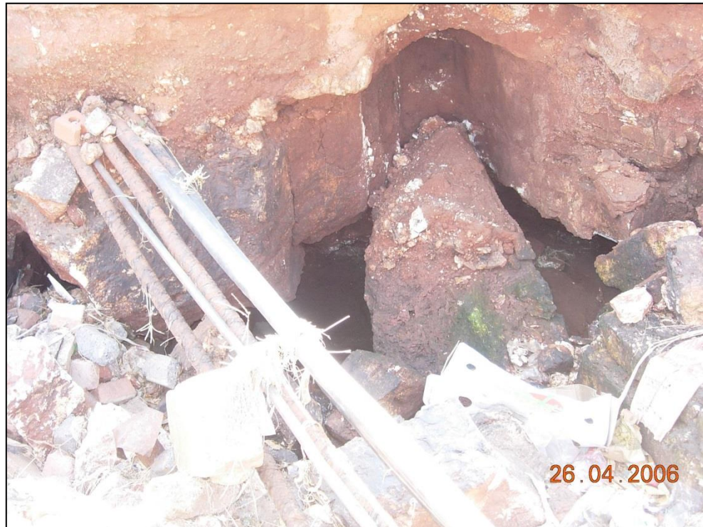
Plate F.2: Cavernous conditions visible between chert boulders in sinkhole area.
