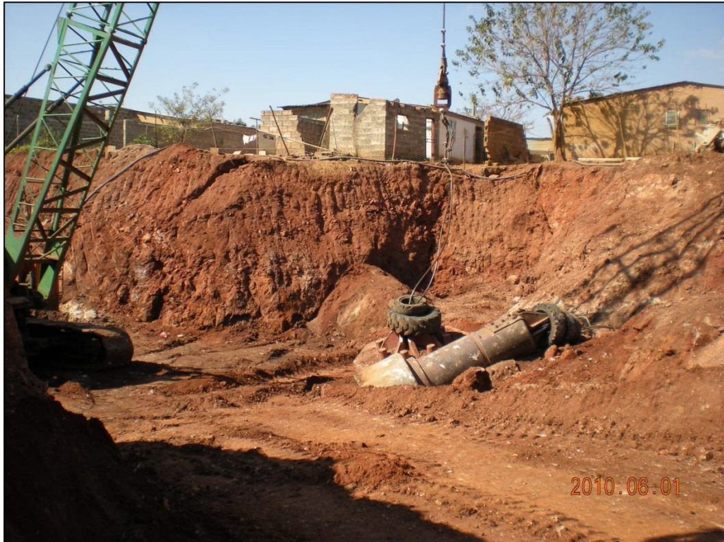
Plate E.5: Dynamic Compaction in progress in affected area at Stands 2655 to 2657.
