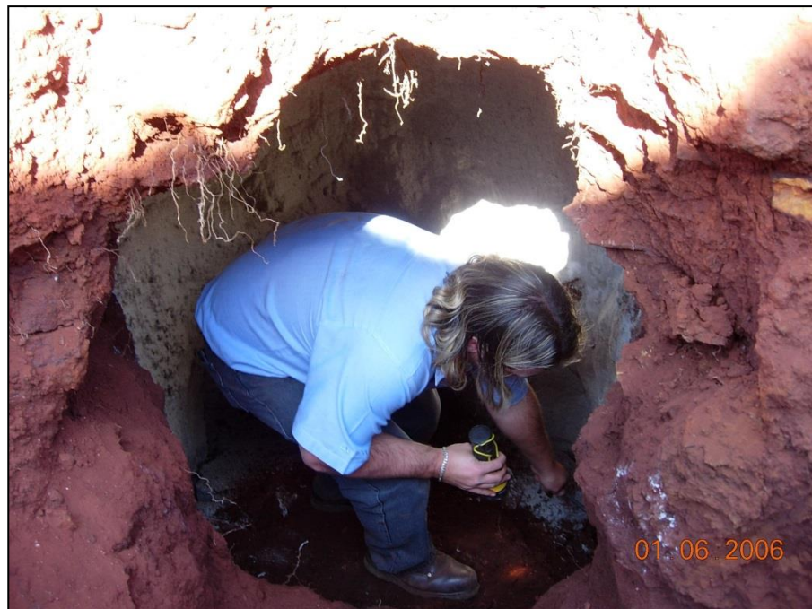
Plate A.3: Cavity encountered in Borehole BH3 and in southern side wall of sewer trench.
