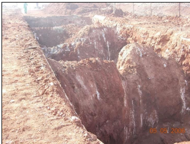
Plate 4: Bulk excavation Bierman Road exposing shallow dolomite bedrock, photo taken towards the east.
