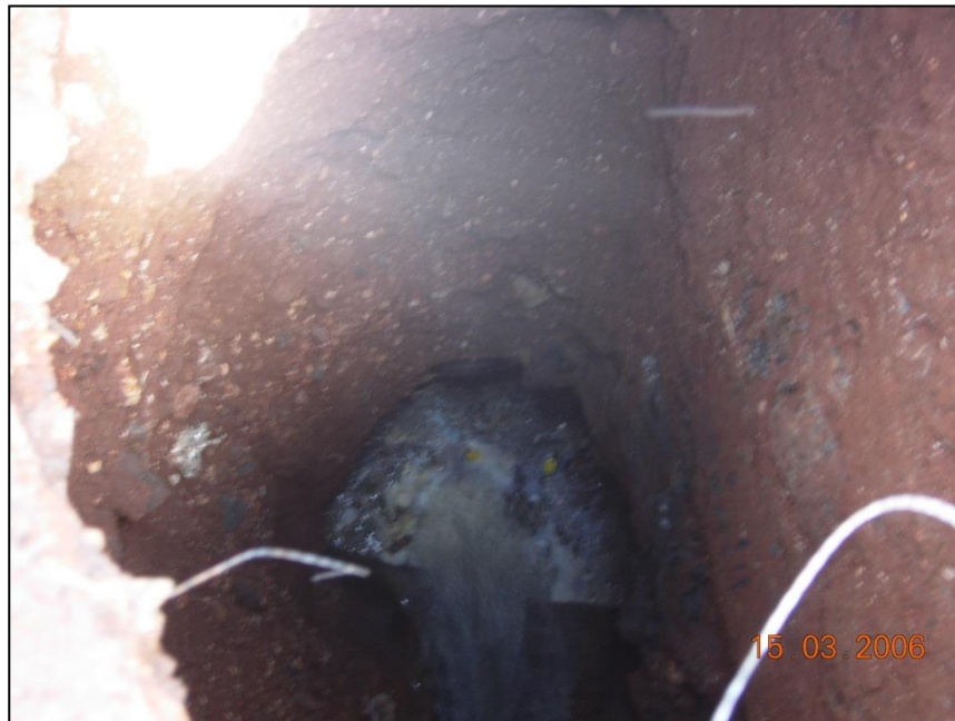
Plate E.2: Broken sewer with fast flowing effluent causing subsurface erosion.
