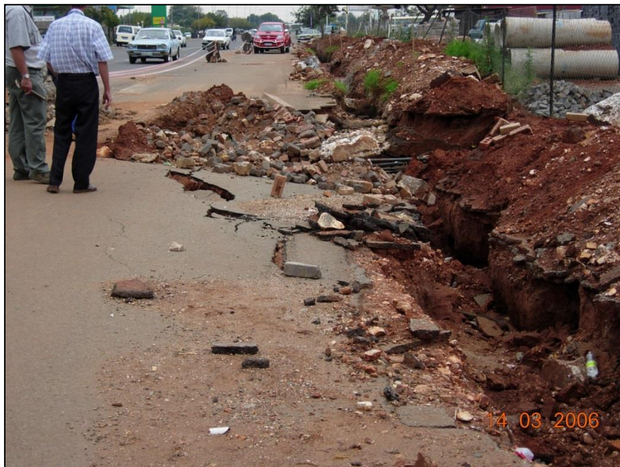
Plate F.1: Sinkhole in south-eastern servitude of M.C. Botha Road.
