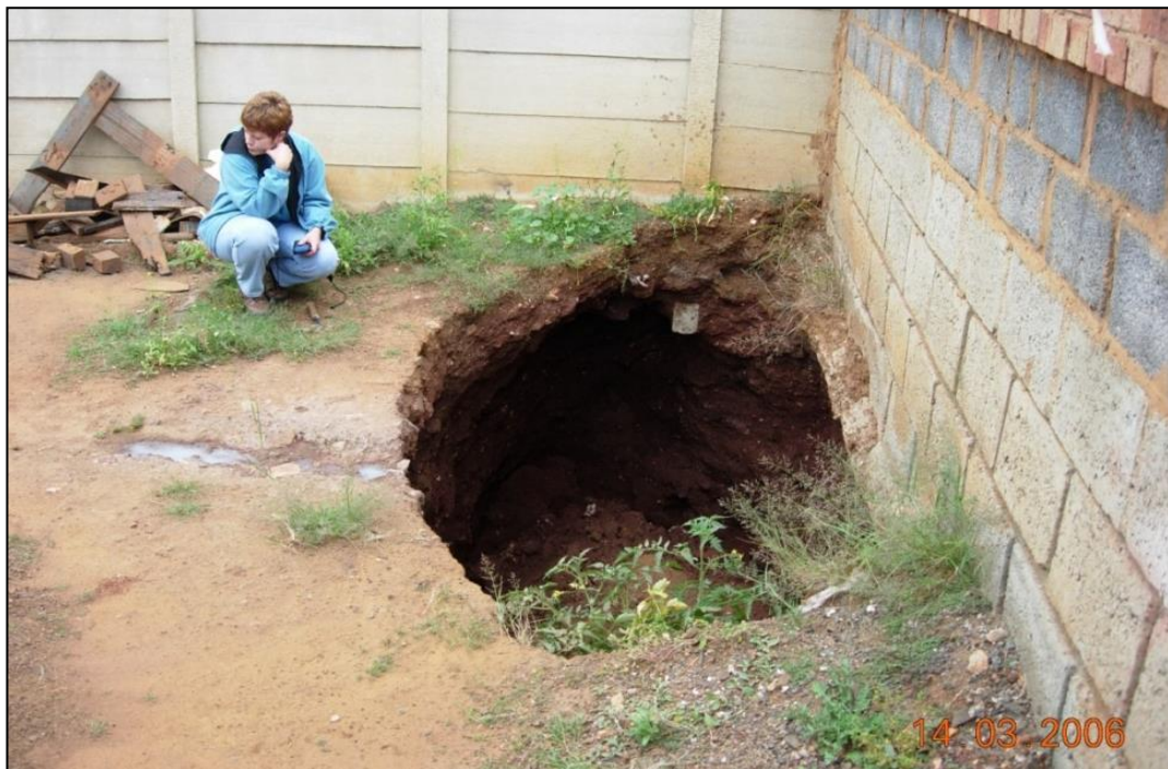
Plate A.1: Sinkhole on Stand 20359.
