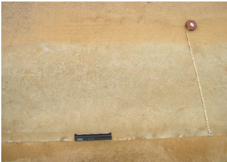
Photo 3: Development of cracks as at 20/01/2005 after 400 000 E80s (View of least cracked portion on Section 4 (50 mm)).
