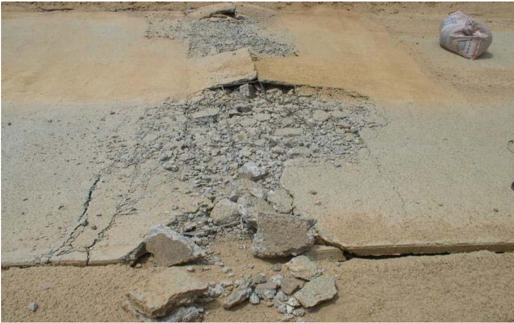
Photo 2: Blow-up in November 2003.
