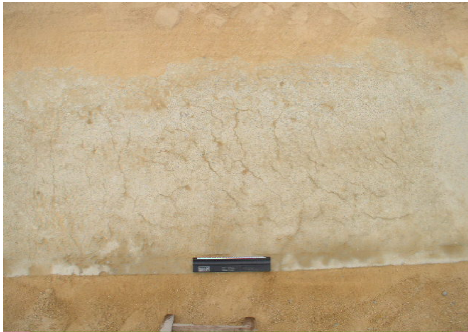
Photo 4: Development of cracks as at 20/01/2005 after 400 000 E80s (View of worst cracked portion Section 4 (50 mm)).
