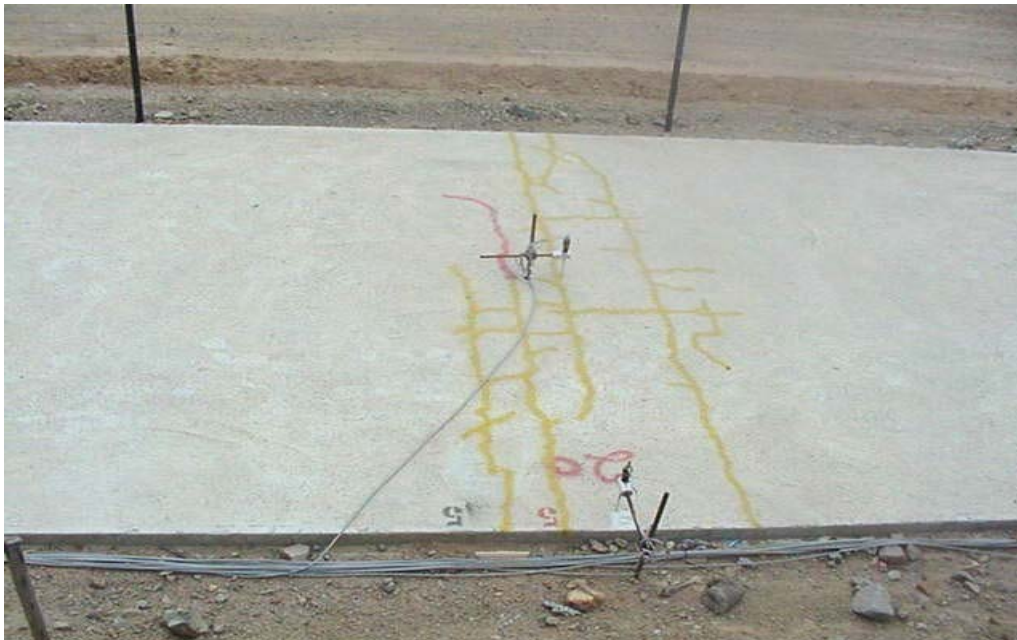
Photo 1: Shrinkage cracks at transition between Sections 4 and 5.
