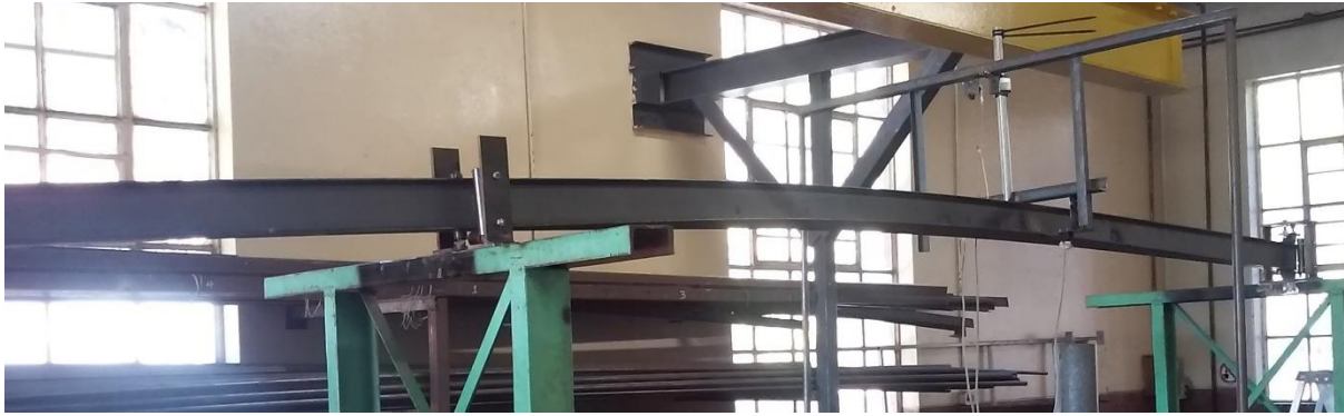
Figure 5.16: Upward deflection of the backspan segment.
