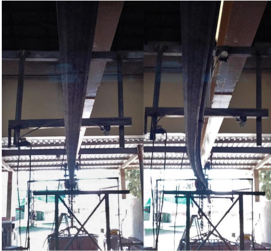
Figure 5.11: Original position (left) and the buckled position (right).
