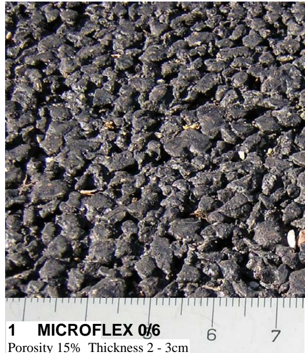
FIGURE 8 Thin, low-noise, porous rubber-bitumen asphalt road surface used in cities and residential suburbs
