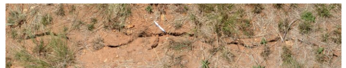
Fig. 3. A portion of an approximately 30 m long tension crack that was observed on the western edge of the deformation feature.
