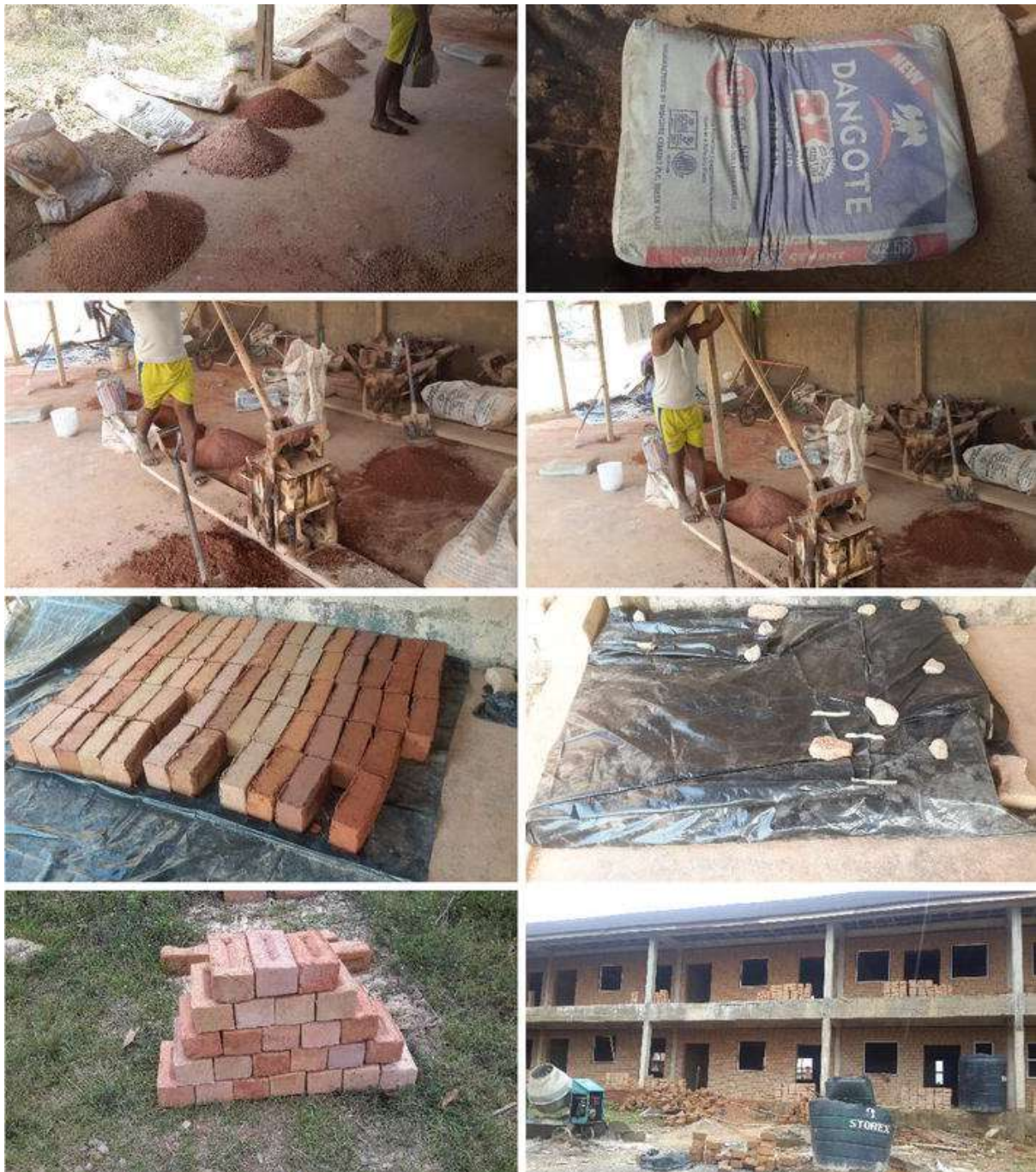
Fig 4: Pictorial description of processes involved in brick making. (starting from soil screening, stabilizer, mixing, compression, curing, stack piling and use)
