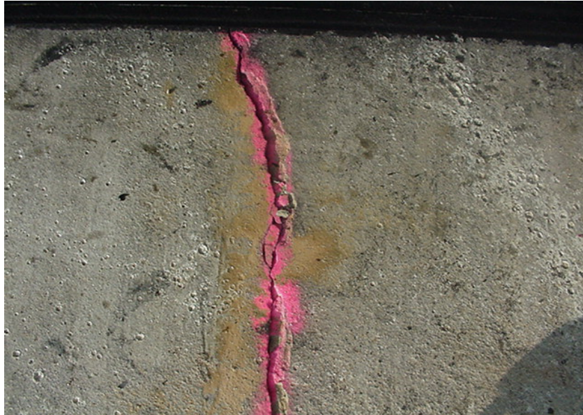
Figure 4. Spalling of a crack as a result of relative vertical movement and pumping.
