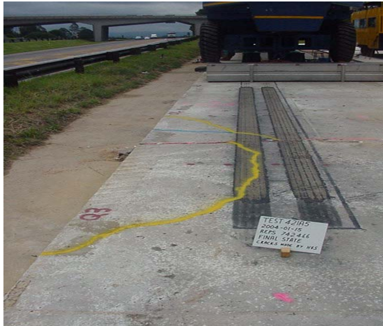
Figure 2. Crack pattern at the end of the test on the undowelled dolerite section.
