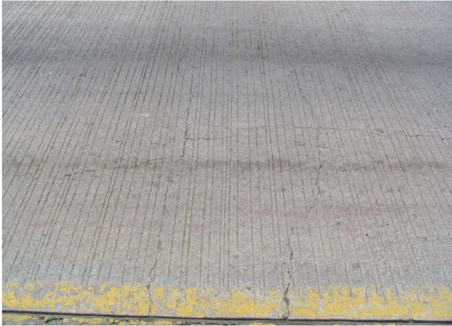
Figure 13. Longitudinal cracks at clustered transverse cracks can lead to punch-outs.
