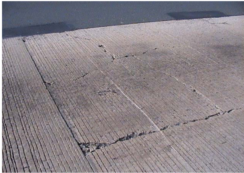
Figure 11. A cluster of cracks at a transverse construction joint and an open edge joint.
