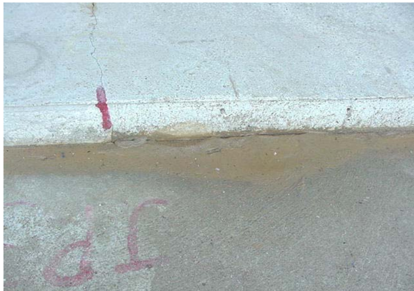
Figure 3. Pumping from under the leave slab, the right hand side of the crack.
