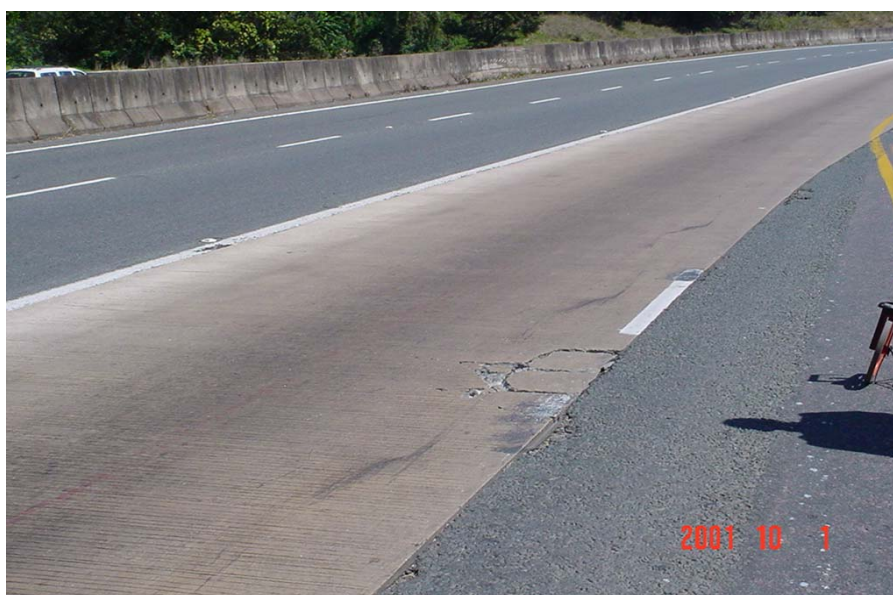
Figure 12. A cluster of cracks, an open edge joint and edge loading lead to a punch-out.
