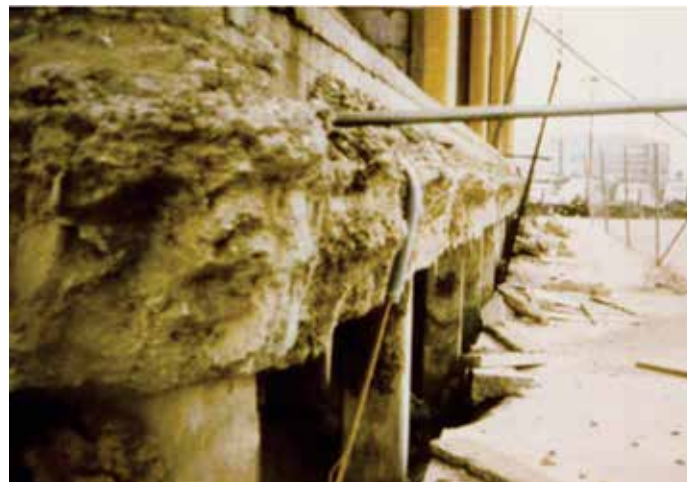
Figure 132 - Shows the waste fill settling away from the building
