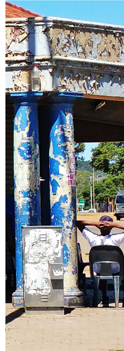
Fig.21. Layers peeling away
