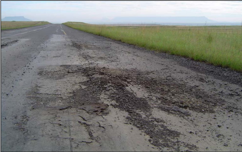
Figure 1: Heavy vehicle overloading contributes to accelerated pavement deterioration, which not only increases the cost of road maintenance (exponentially) but also increases vehicle operating costs.
