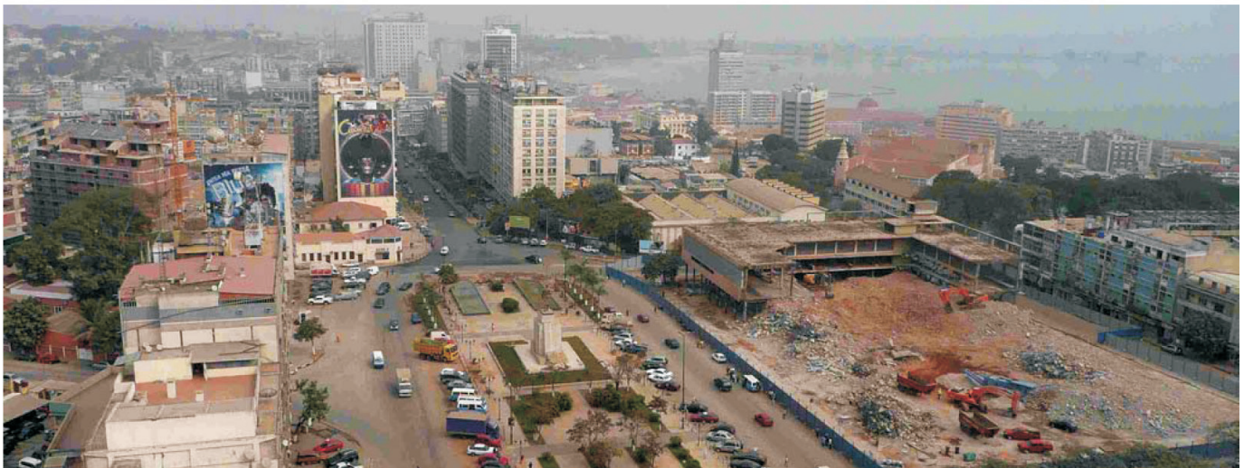
PERSPECTIVE OF LUANDA CITY, in 2008, showing the demolition of Kinaxixe Market designed by Vasco Vieira da Costa. It was considered to be one of the most relevant testimonies of modernism's achievements in Africa. It will be replaced by a commercial and residential development.
