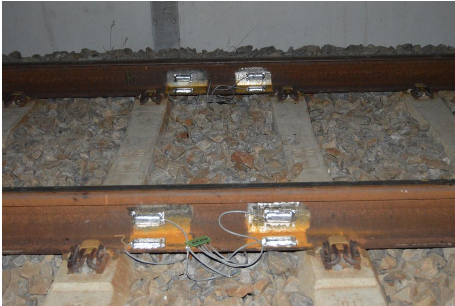
Figure 3.24: Encapsulated Strain Gauges Covered in Permanently Plastic Putty with Aluminium Foil (ABM75)
