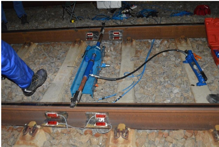
Figure 3.26: Original Set Up of the Calibration Rig for the Lateral Strain Gauges
