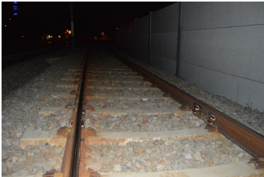
Figure 3.20: Longitudinal View of Installed Encapsulated Strain Gauges
