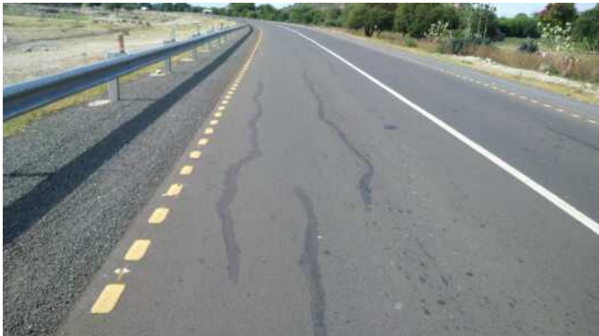
Figure 1: Typical longitudinal cracking on Project A
