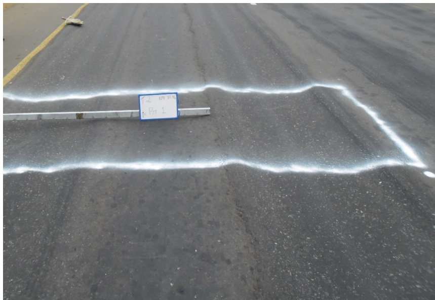
Figure 2: Extent of rutting on Project B
