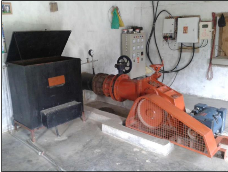
Figure 2-66 - All the components of the hydropower plant in the turbine room (Turbine, generator, electrical control panel and ballast load)
