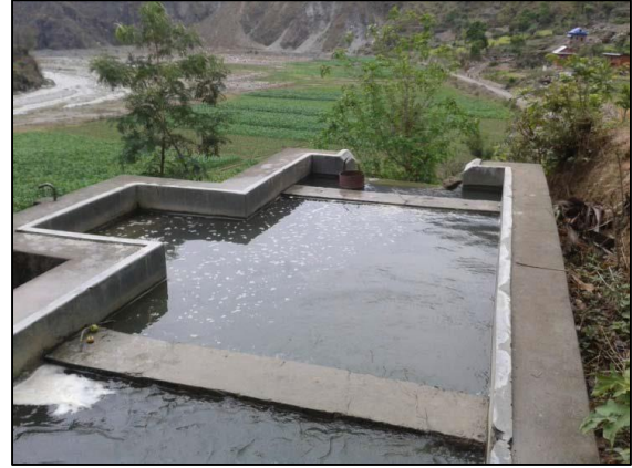
Figure 2-64 - Intake collecting water from stream
