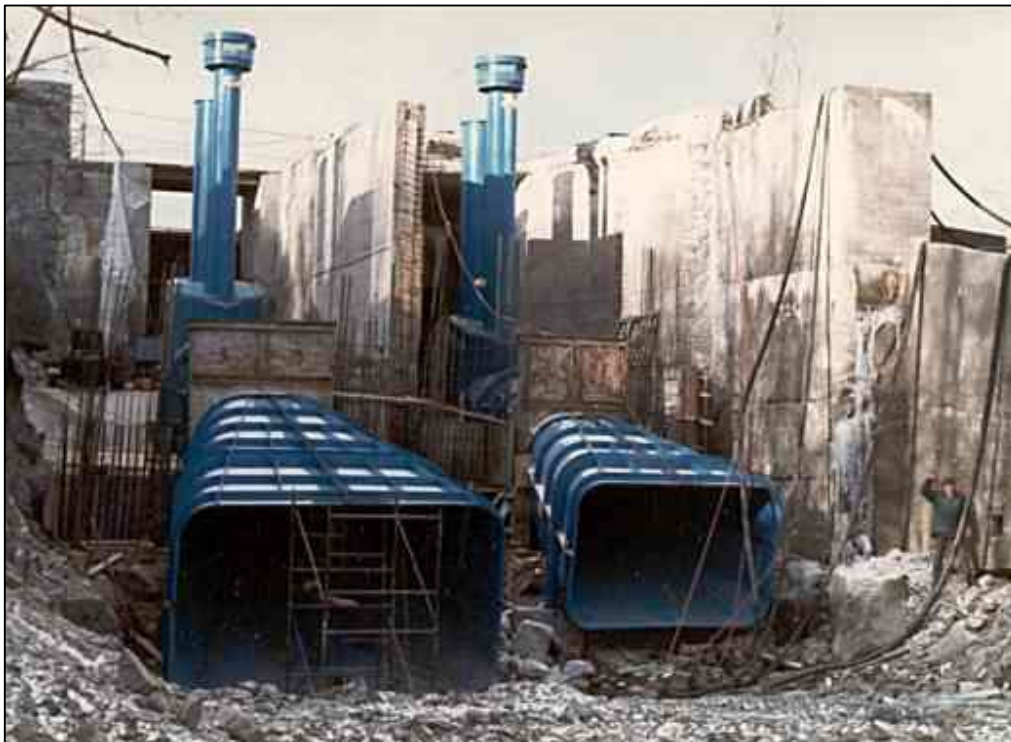
Figure 2-28 - Bulb turbines and draft tubes - Sebec Hydropower plant (Swiftriverhydro, 2015)
