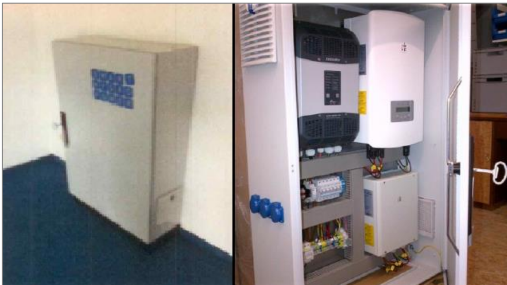
Figure 5-86 - Kinetic Turbine Controls (Smart Hydro Power)
