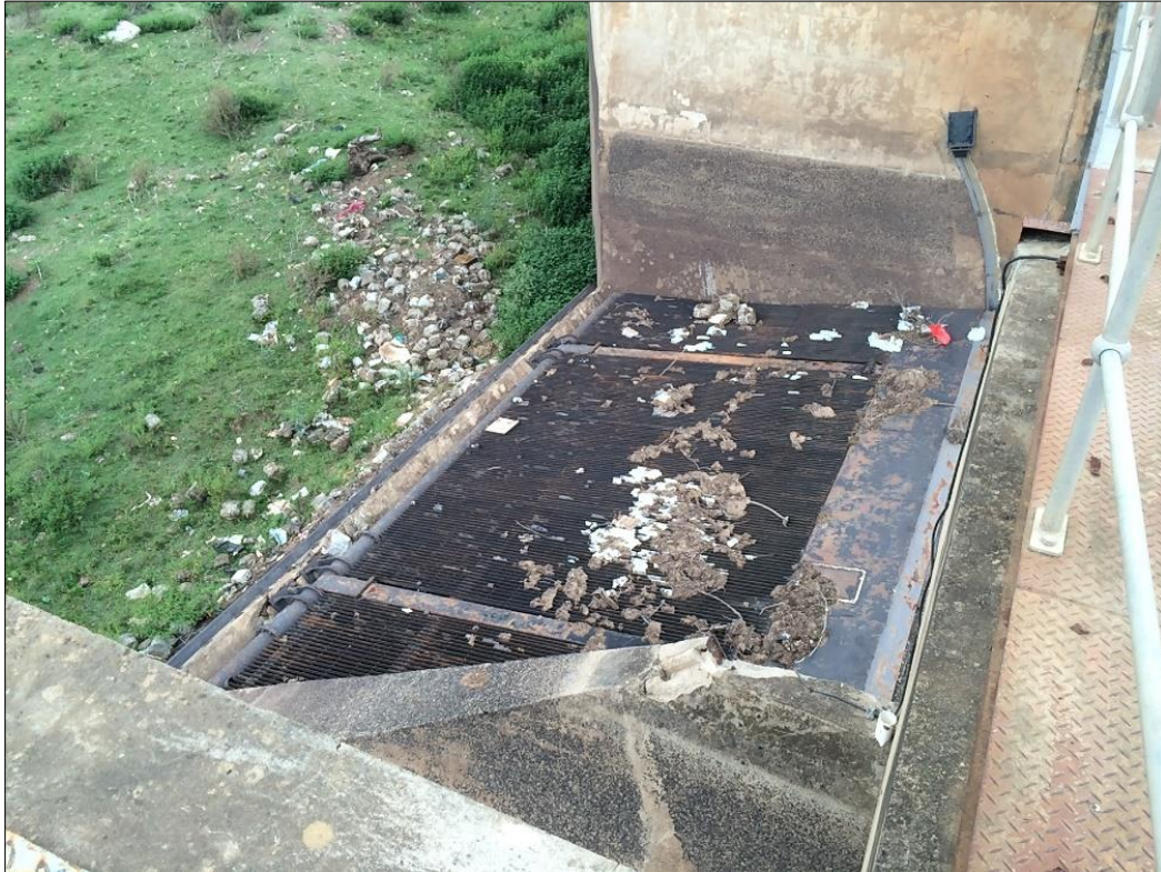
Figure 2-59 - Intake grill/screen with debris – First Falls Hydropower Plant, Mthatha River
