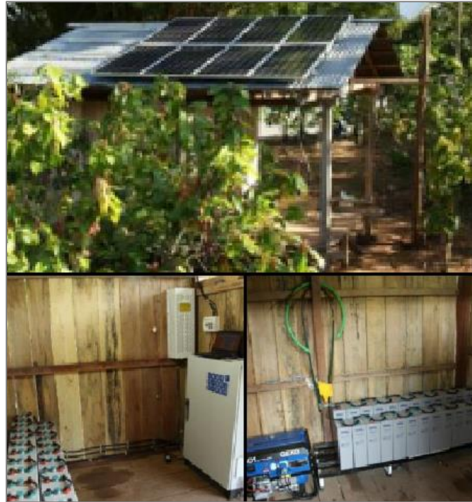
Figure 5-87 - Control Room (Smart Hydro Power)
