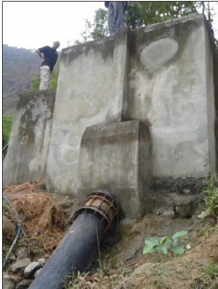
Figure 2-65 - Penstock supplying water to turbine room
