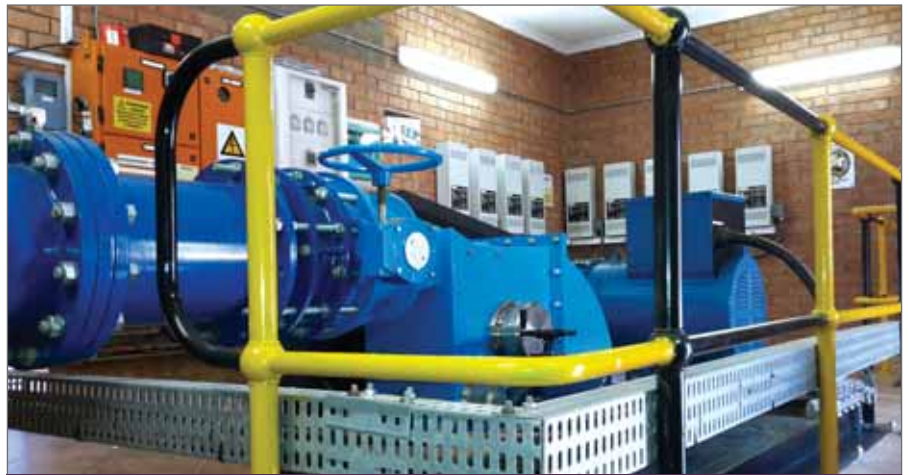
Figure 3: Banki turbine installation at Bloemwater's Brandkop Reservoir
