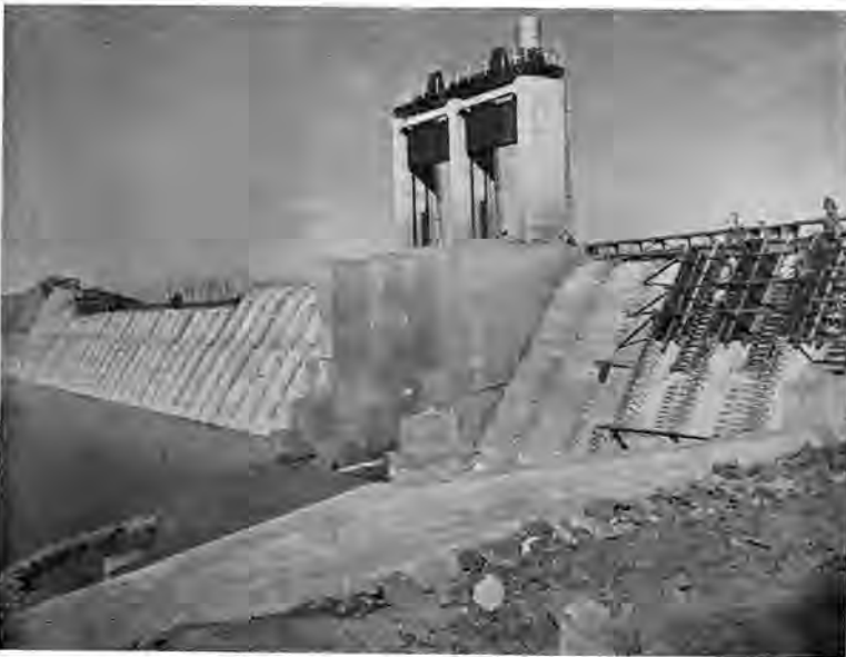
The works in the process of construction, with siphons in various stages of completion, the first battery of three being ready for operation.
