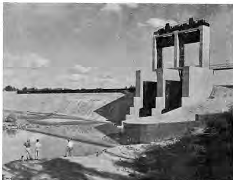
The original works before alterations, showing gravity section weir with automatic trip falling shutters, 5 ft. 6 ins. high, mounted on the crest.
