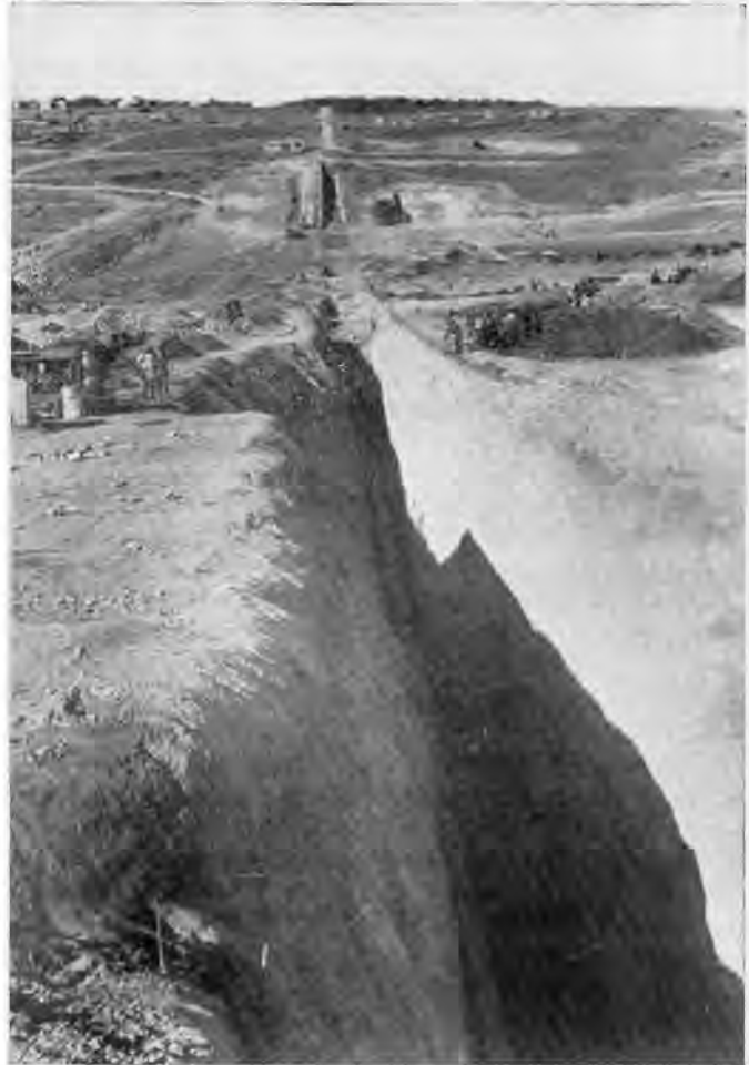
The Rooikrantz Dam site, looking north. Along the centre-line a trench has been excavated down to rock.
