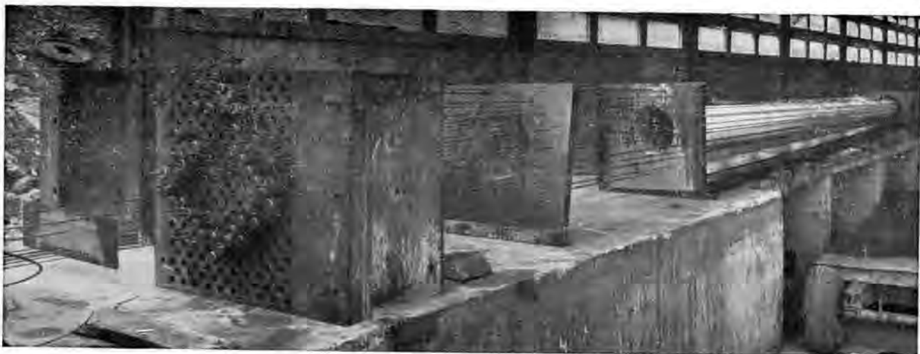
Anchor on short casting bench, showing wires and cores in place for hollow columns for single-storey building.
