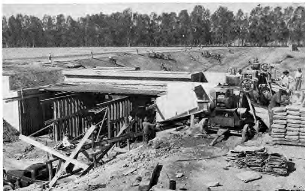
The central concrete batching plant with the concrete bridge in the background. The subway will become the main entrance to the workshops from the Pretoria side.
