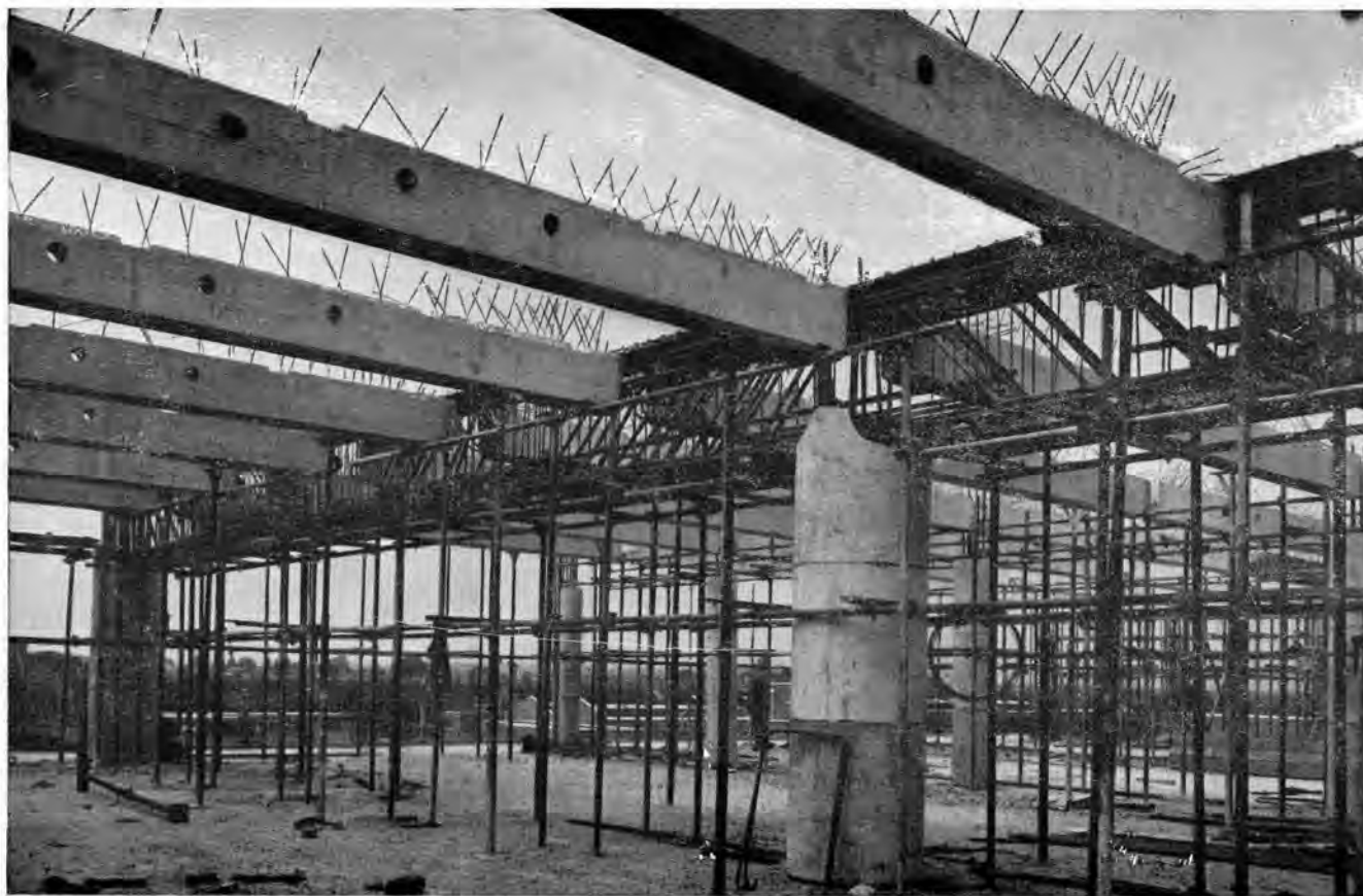
Pre-stressed pre-cast secondary beams erected ready for the casting of the main beams at a new paint factory.
