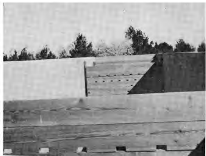
Inside of the sedimentation tank with the wooden baffles in position.
