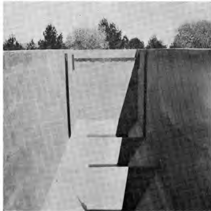
Interior of the sedimentation tank without the baffles in position.
