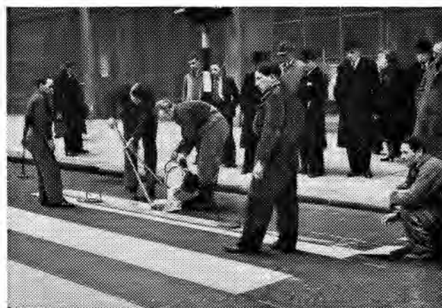
Fifty-one new-type safety crossings have been laid in the Borough of Westminster, London. The road is sprayed with an adhesive on to which strips of plastic are laid. At least a year's wear is claimed from the plastic material.
