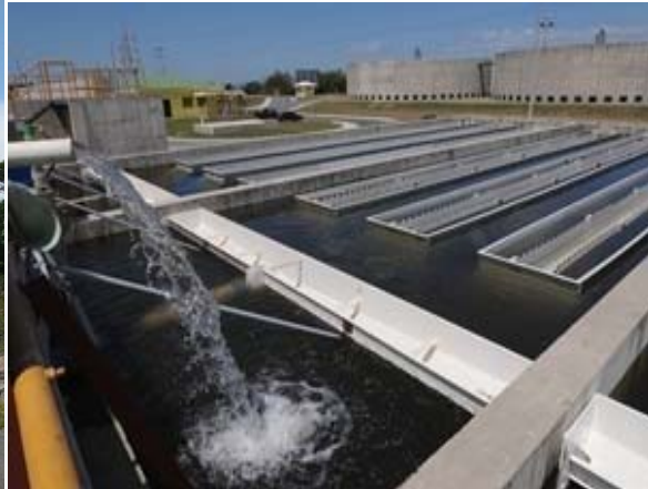
Fig 2: Bushmead water treatment plant
