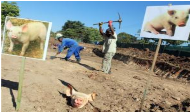
Figure 2: A pig's head thrown on the site where a mosque is being built in Kwa-Zulu Natal
