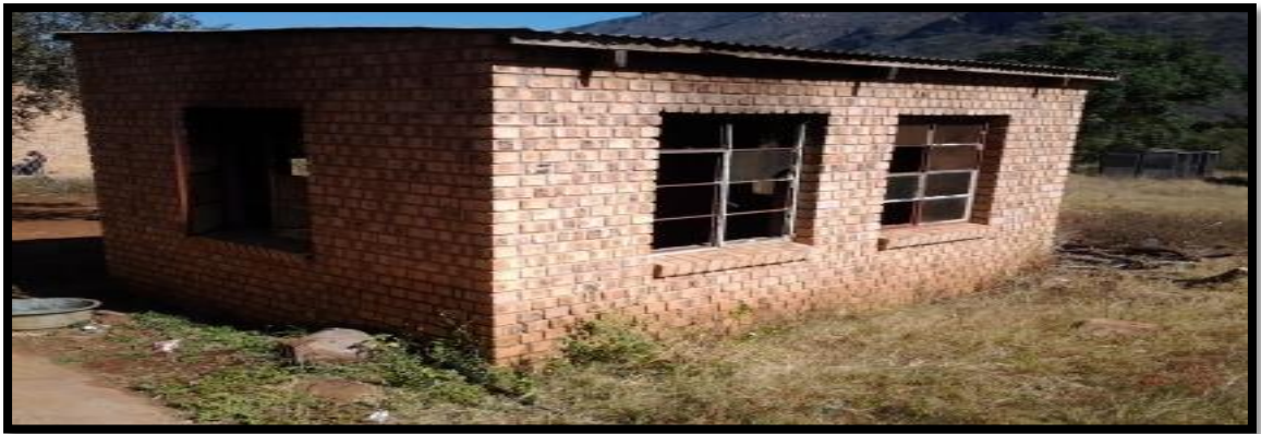
Photo 12: Kitchen at School B
