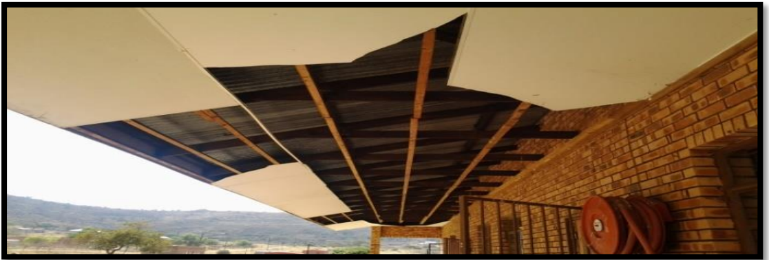
Photos 4 and 5: Holes in the ceiling at School A
