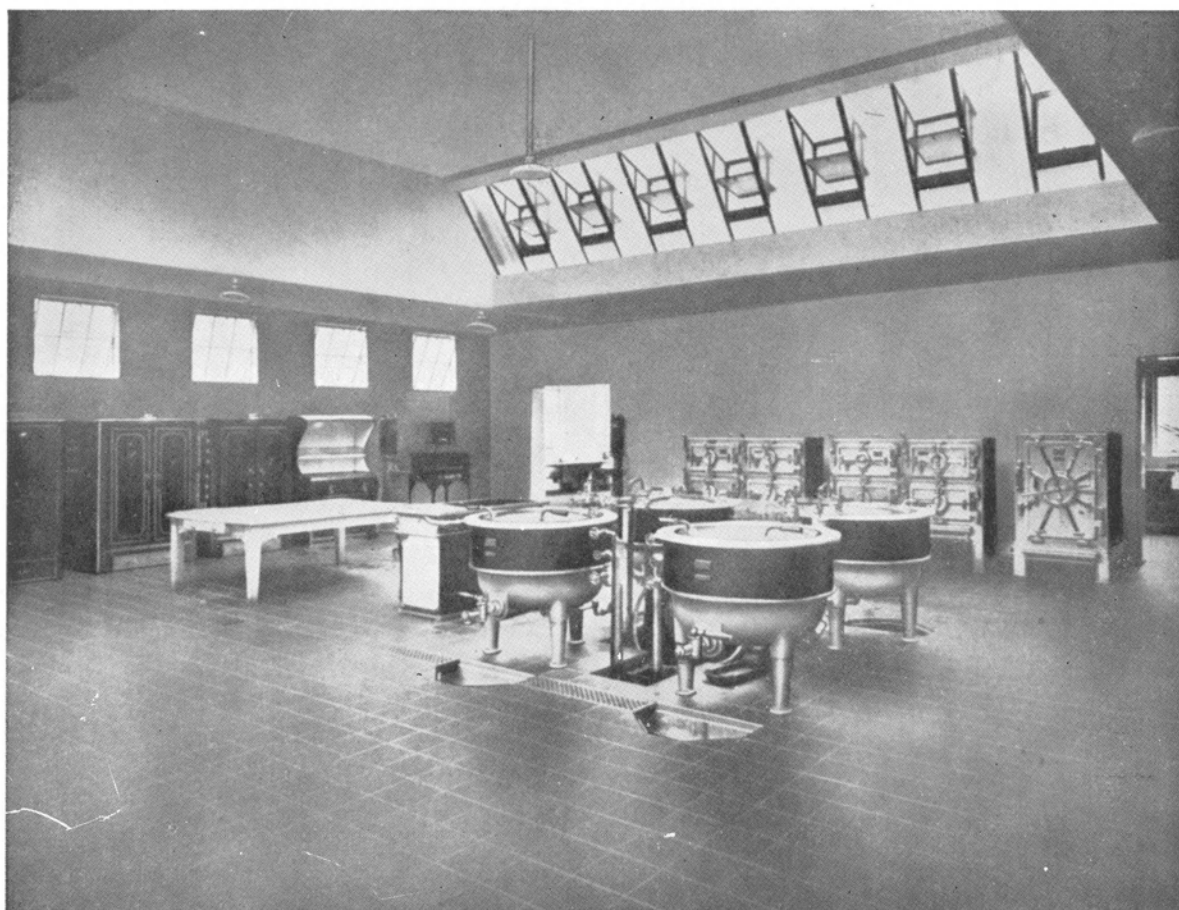
The photograph above shows typical Ashwell & Nesbit equipment recently installed in a modern Kitchen of a large hospital. The apparatus is finished in grey mottled enamel.
