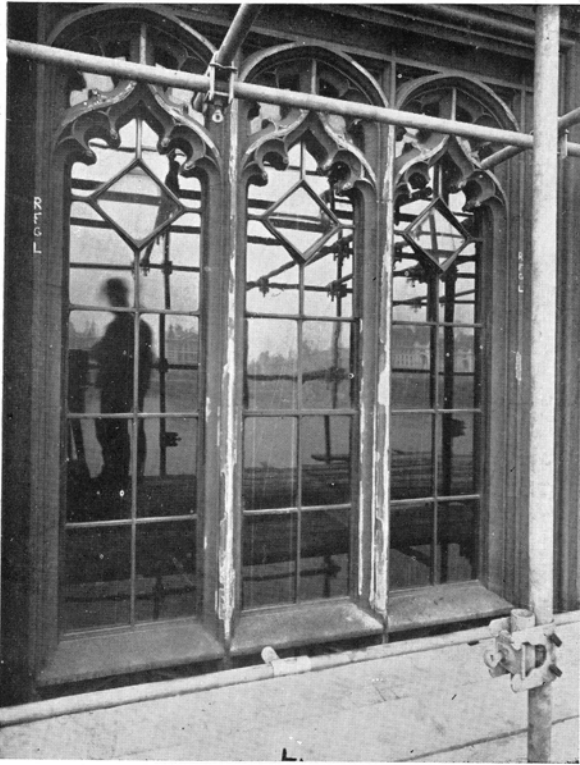
A window: Note the surface decay on the face-bedded mullions.
