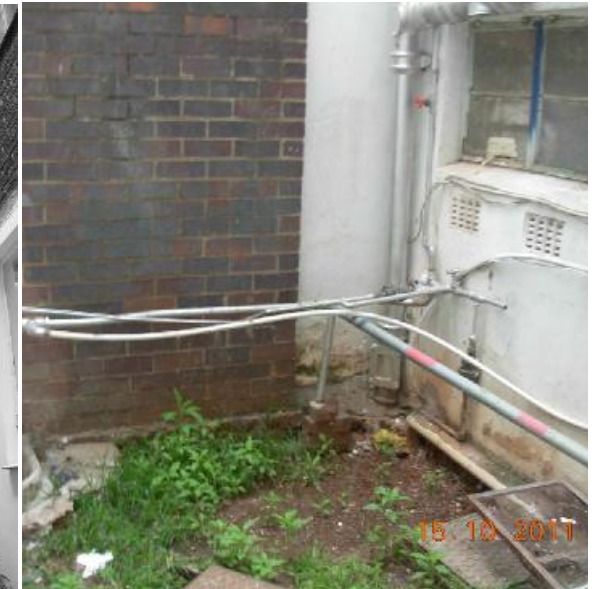
Figure 2.39 Internal service duct
