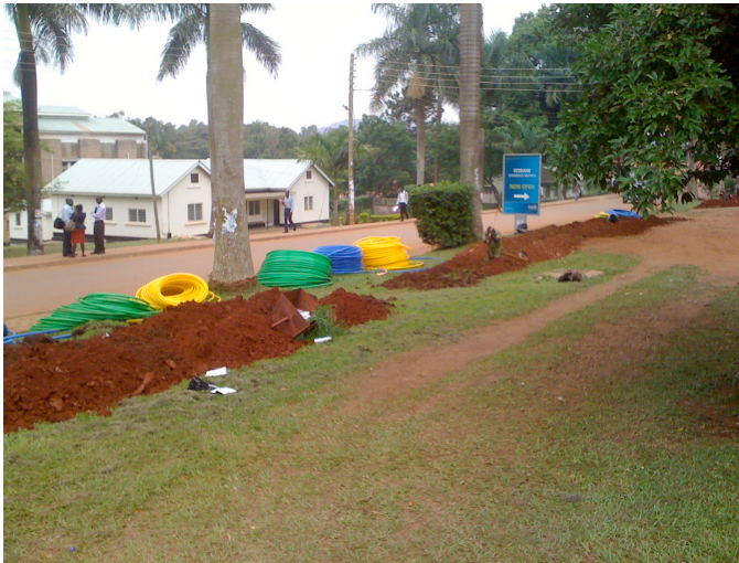
Figure 12: The laying of Internet Cables near the French Department (Photo by RSB)
