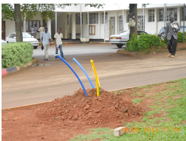
Figure 13: Optical fibre cables termination near the Faculty of Arts and Social Sciences (Photo by RSB)
