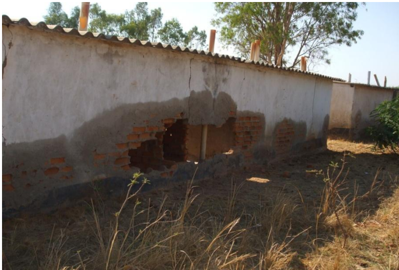
Picture 6: The state of toilets at Kakora Primary School
