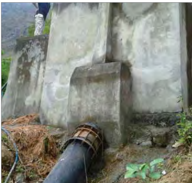
Figure 4: Penstock supplying water to turbine room
