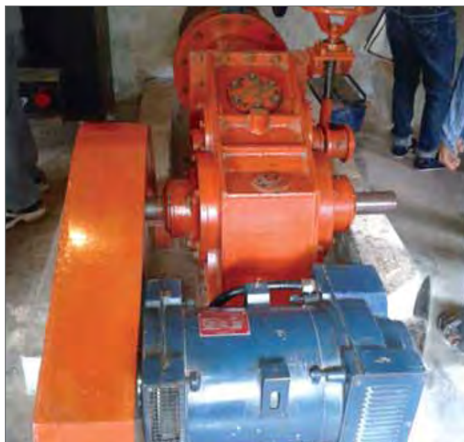
Figure 5: Cross-flow turbine and generator
