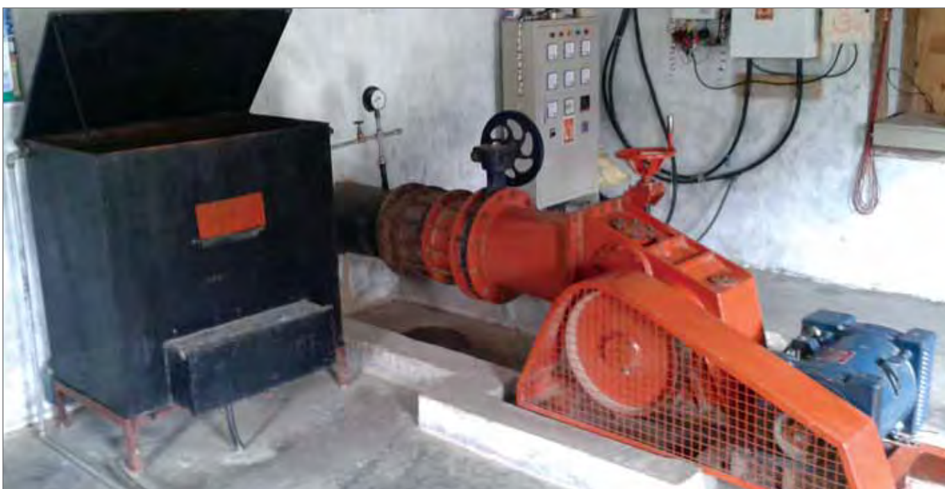
Figure 6: All the components of the hydropower plant in the turbine room (turbine, generator, electrical control panel and dumb load)
