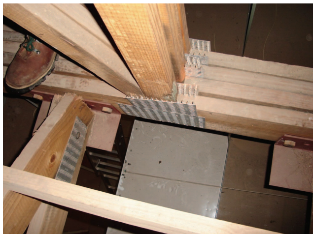
Figure 3. This shows the outer ply loading of a multiple ply girder truss and tensile failure (nail plate pulling out)
