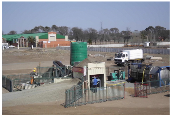
Figure 6: Pug mill at site plant.
