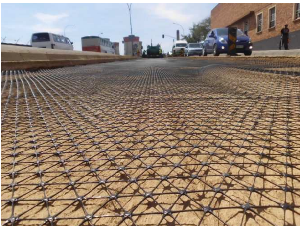
Figure 3: Rolled out Triax TX170.
