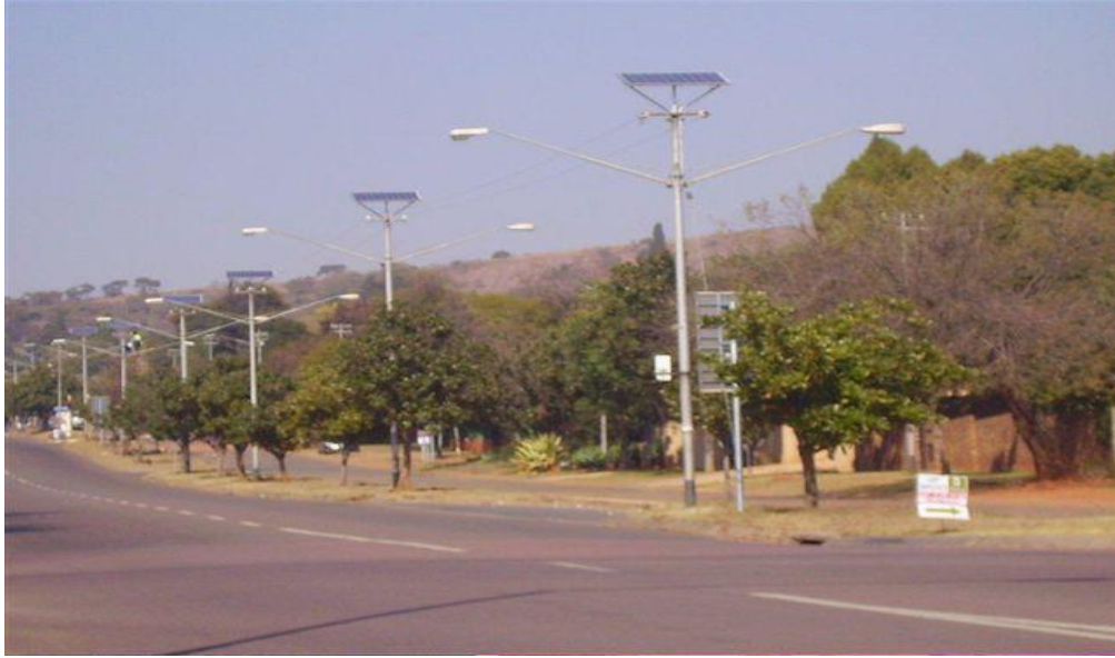
Figure 3.4: Street lights fitted with solar panels along Queen Wilhemina Street, Brooklyn
