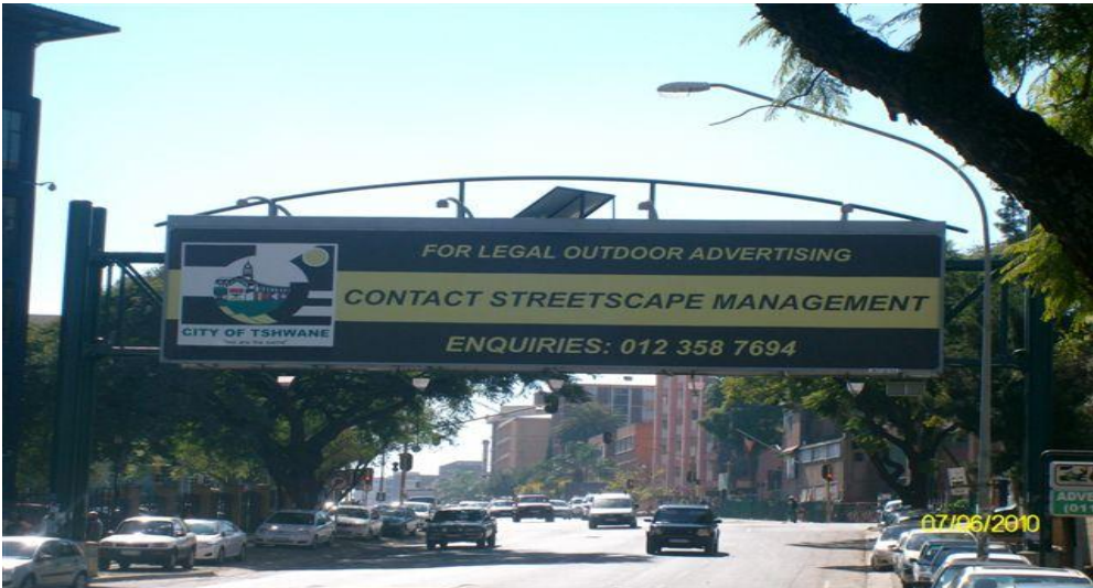
Figure 3.3: Retrofitted Billboard operating by solar energy – Corner Troye and park Streets (Arcardia)
