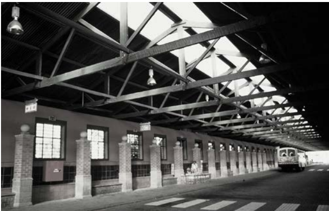
Fig.5.10: Interior view of polycarbonate sheeting inserted along the length of the roof to allow admittance of natural light (Marnus Barnard).
