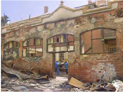
[Fig. 46] Damage caused by the fire
