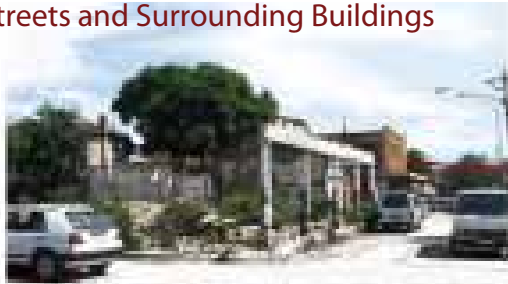
Figure 6.3.a Half demolished structure corner of 7th and Grand Street. See brick and plaster material use (Author, 2010).
