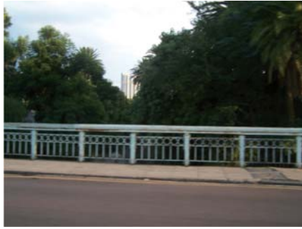
Figure 7.5.8. Lions Bridge crossing the Apies River along Church Street (Author,2011). The bridge marks the important crossing point between Sunnyside and The CBD as well it sits on the major east west axis of Pretoria.
