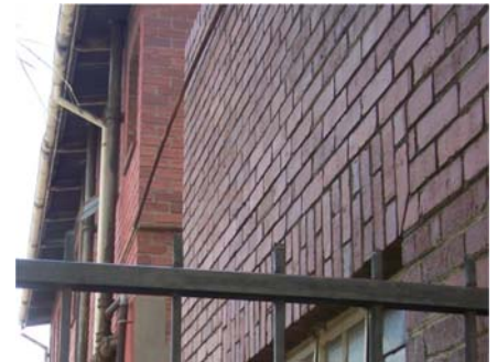
Figure B. 41 E - stand 1183 (Author, 2011). Description : outbuilding/store User : Arcadia glass and frame work (automotive) Analysis : out of scale with the surrounding building scale. building blocks new access of street though the precinct Intervention : could form threshold between open spaces and into main open space
