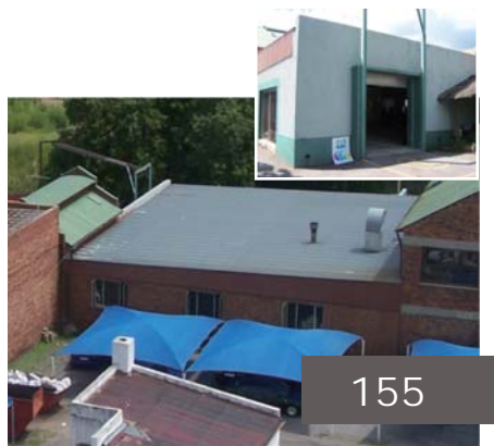
Figure B. 15 & Figure B. 16 B - stand 1053 (Author, 2011). Description : Workshop User : Automotive Analysis : connection between two buildings, detracts from impact two buildings have on the precinct character. Intervention : to be broken open to create entrance into the precinct.
